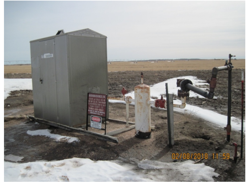
2. Meter shed and Vertical gas separator 50% buried
