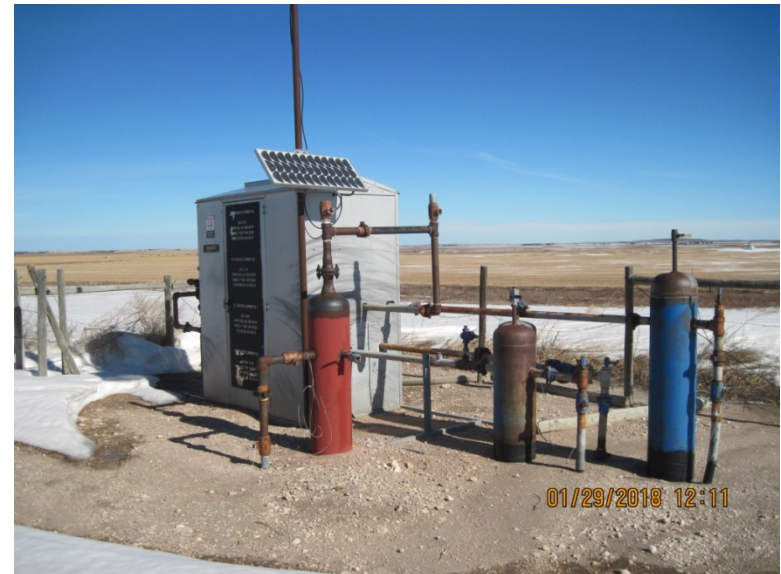
2. Vertical gas separators 50% buried
