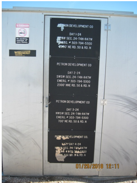
1. Lease signs on meter shed at central battery
