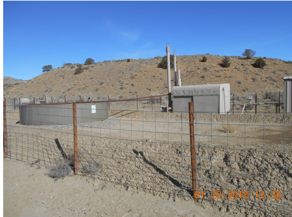
Tank battery with earth berms
