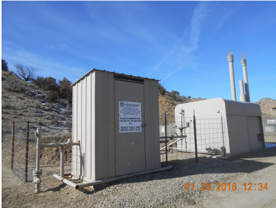
Meter housing with sign and separator
