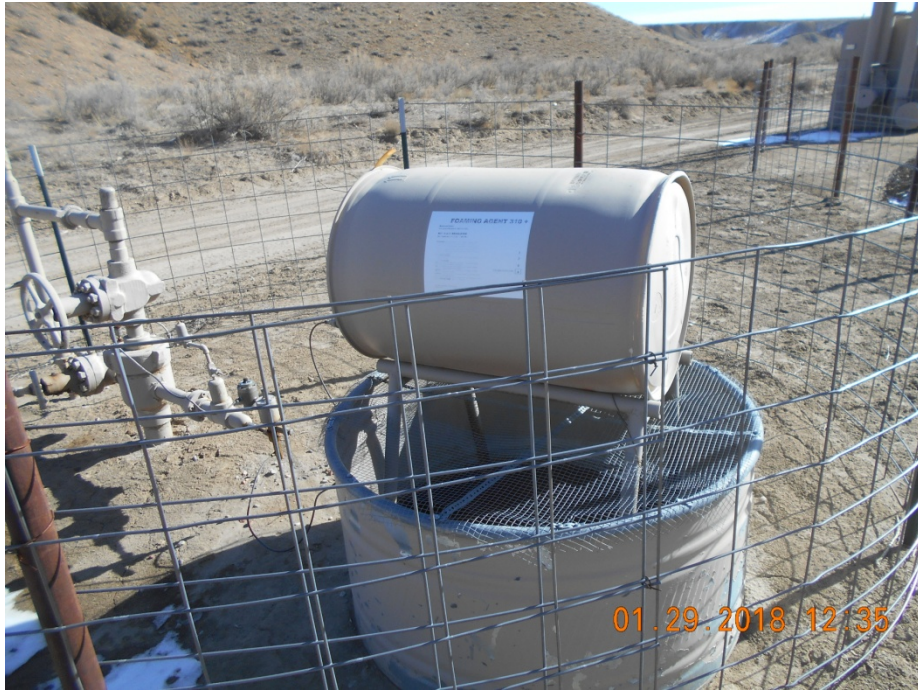
Chemical tank with secondary containment
