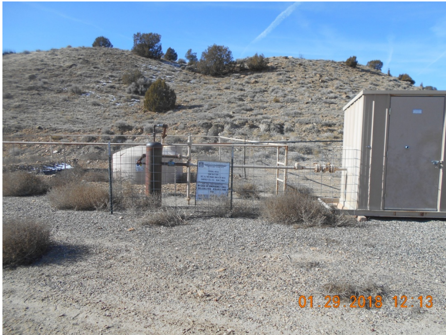
Meter housing and tank
