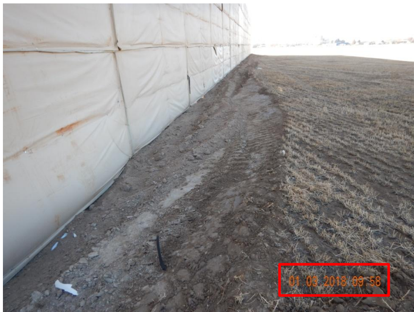
Photo 3. Photo taken from the cut slope of the northern location on January 3, 2018, facing West. Operator has failed to install stormwater BMPs per Rule 1002.f.(2).
