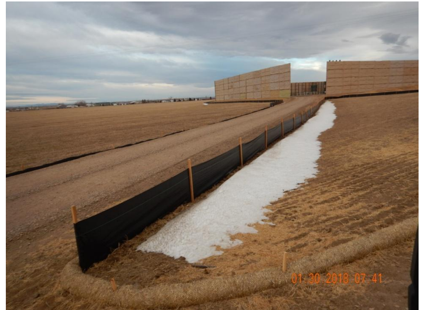
Photo 2. Photo taken east of the location, facing West. Operator has installed silt fence and wattle BMPs around the access road and well location.
