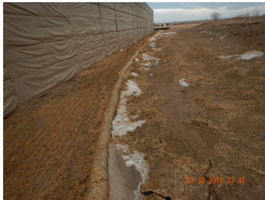
Photo 4. Photo taken from the cut slope of the northern location on January 30, 2018, facing West. Operator has installed straw wattle BMPs along the northern location to control for potential run-on onto location. In addition, the disturbance areas have been crimped with straw mulch.
