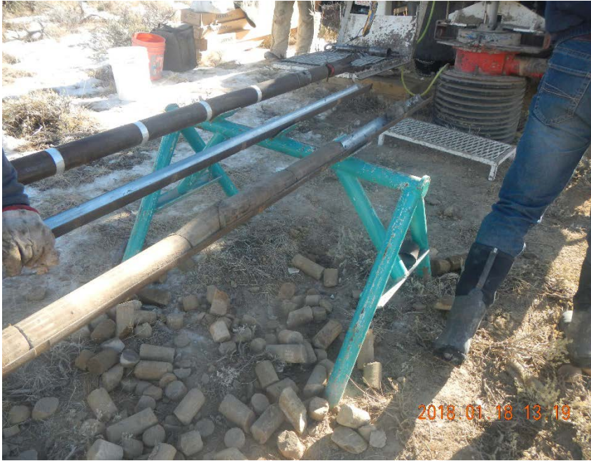
Drilling MW-22. Cores show mostly sandstone. Mudstone was identified by LTE personnel at around 180 ft.
