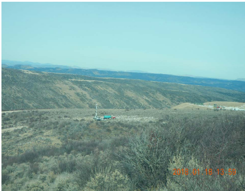
Rig drilling MW-22. Seen from the location of MW-20, looking north northwest. MW-22 is located approximately 2000 ft north northwest of the release point (on Divide Rd.)
