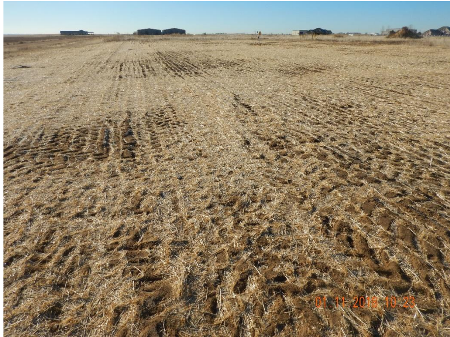
Photo 1: Photo taken from the northeast corner of the former tank battery location, facing south. Photo shows reclamation in-process.
