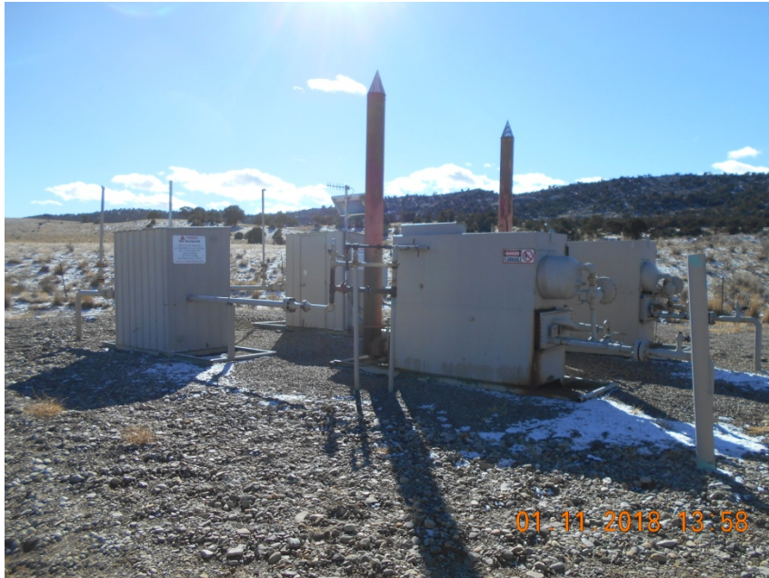
Separators and meter housings
