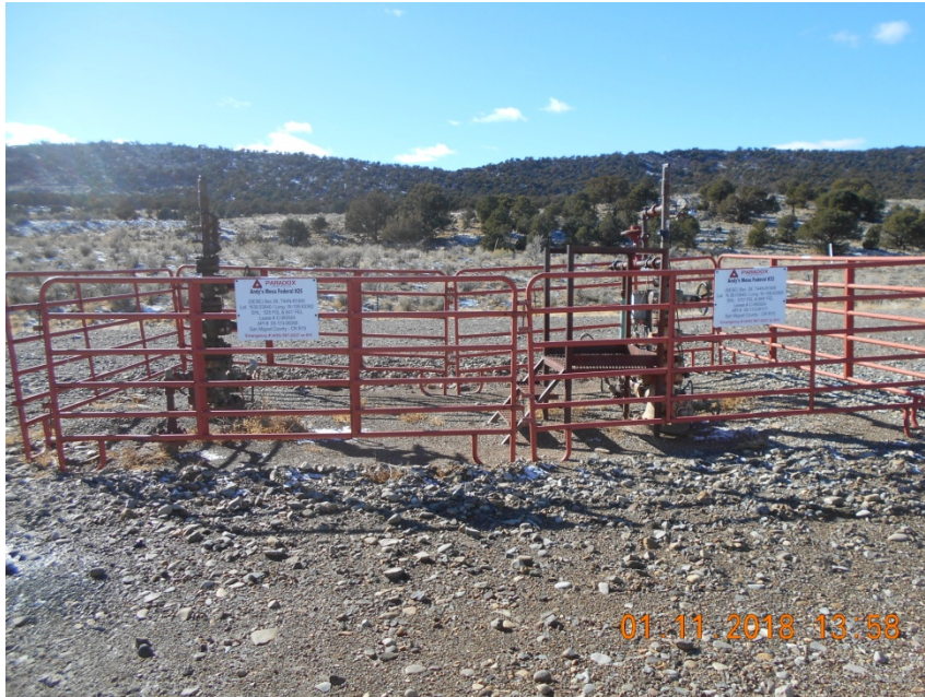
Wellheads with fencing
