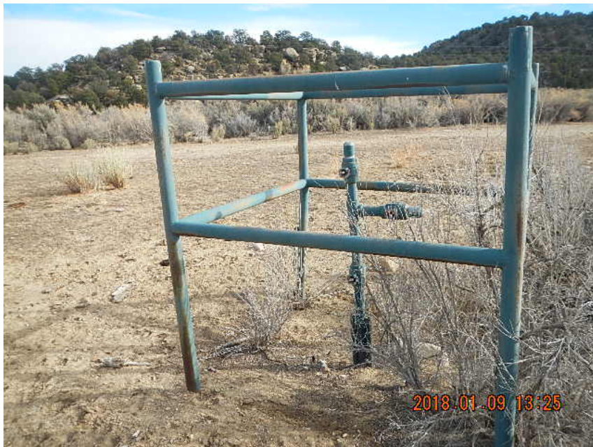
Risers not marked or LOTO
