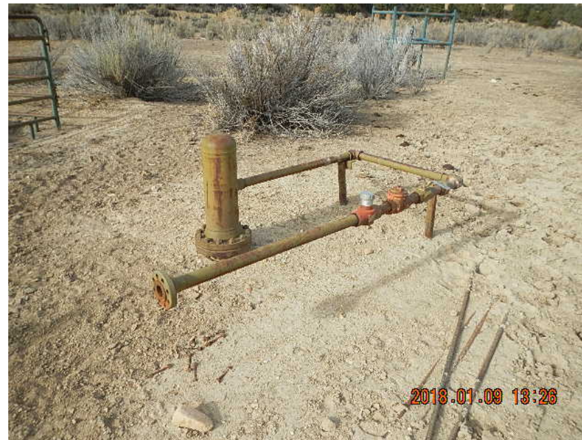
Risers not marked or LOTO
