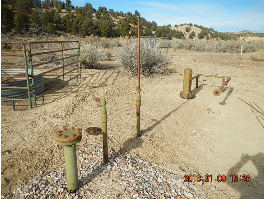
Risers not marked or LOTO
