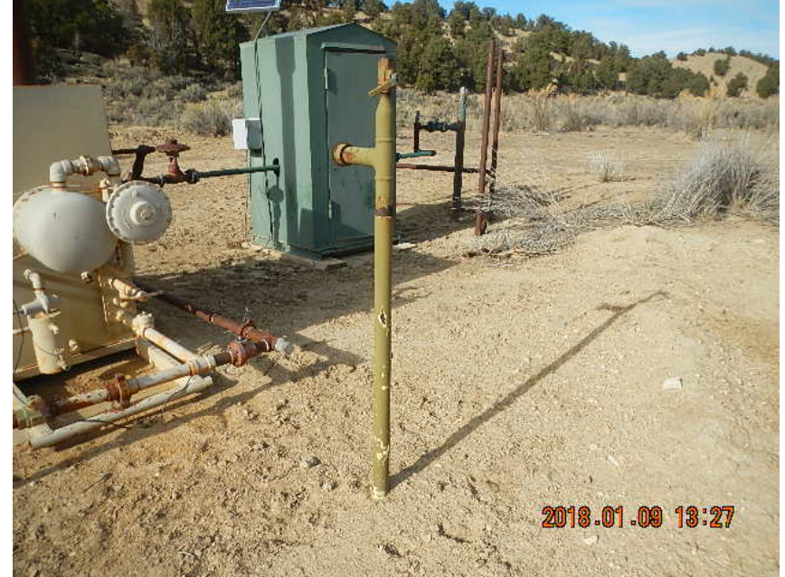
Risers not marked or LOTO
