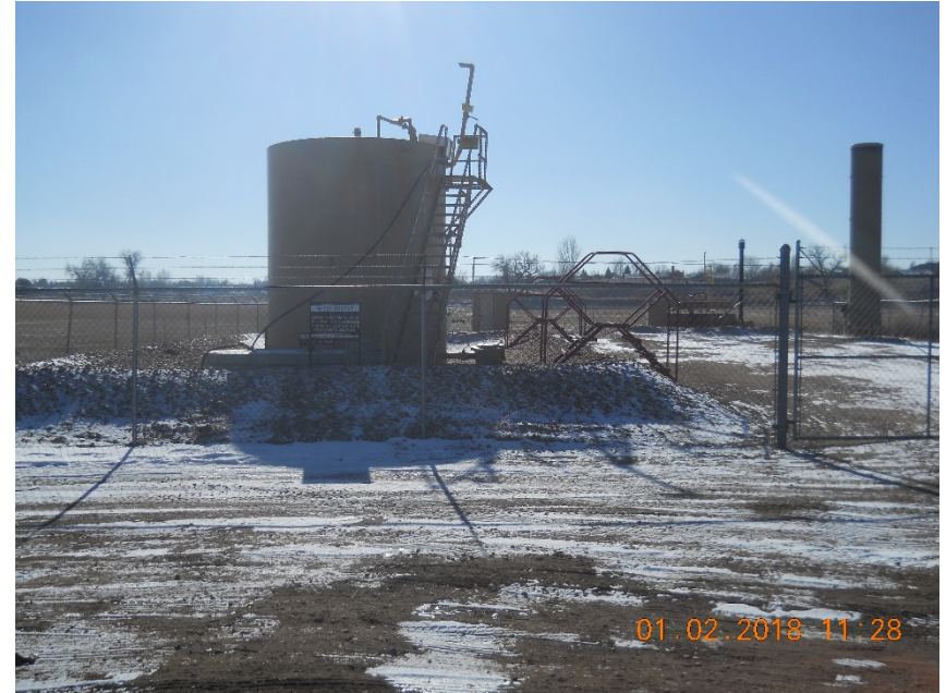
Battery looking south. Trash at entrance of location has been removed
