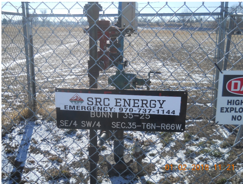
Wellhead looking south. Wellhead sign has been updated with correct operator information/emergency contact number
