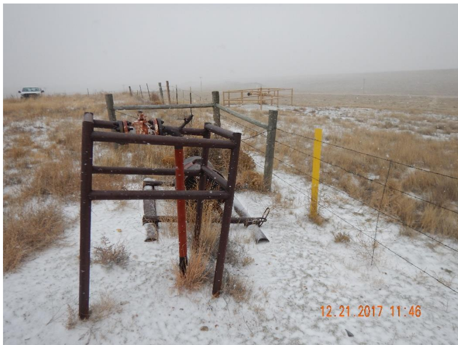
Photo 3: Photo taken from the south end of the location, facing east. Photo shows pipe riser remaining on location.
