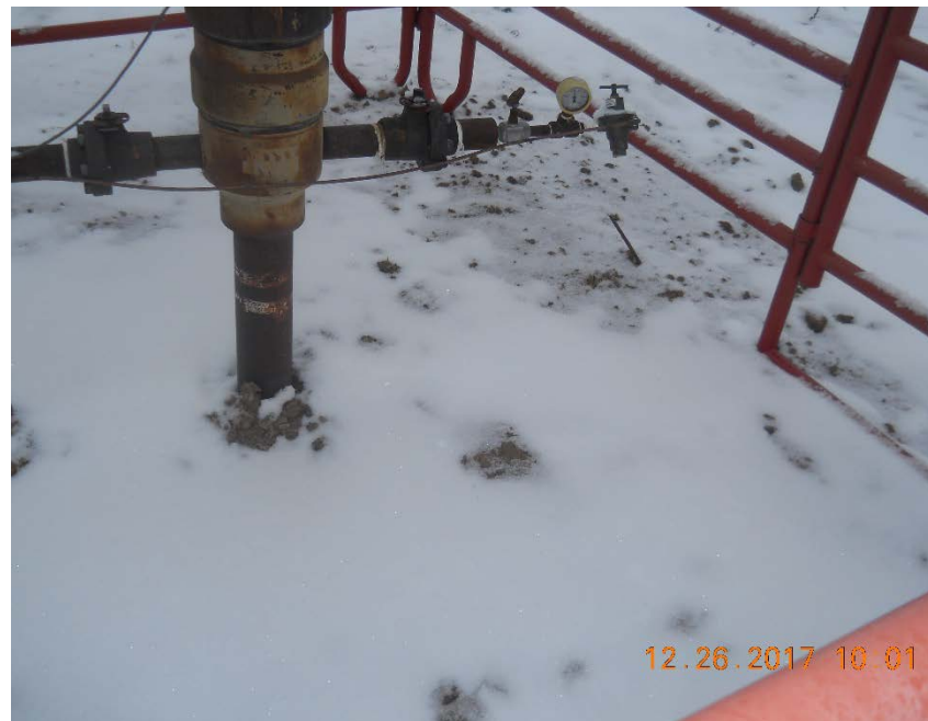
1" steel riser has been cut/capped below surface
