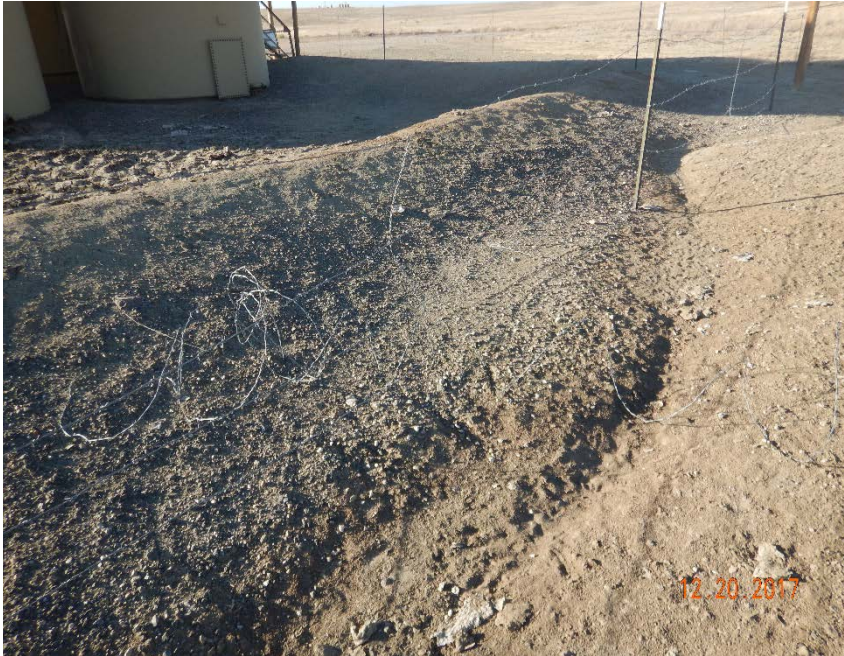
Photo #7 – Damaged fence on north side of battery.
