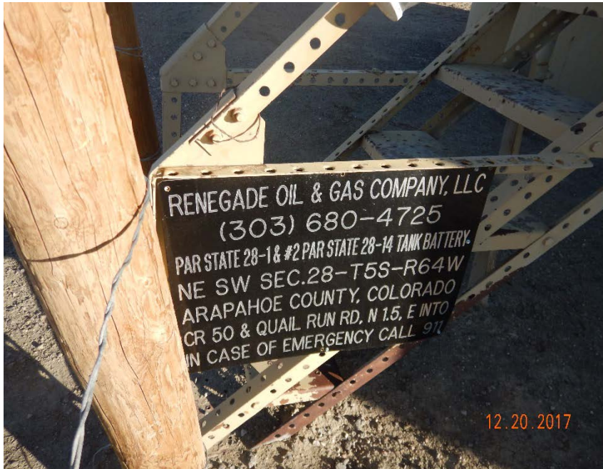
Photo #5 – Battery sign.
