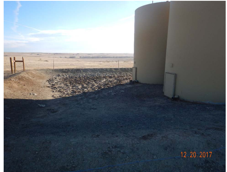
Photo #6 – Shallow berm at NE corner of battery.
