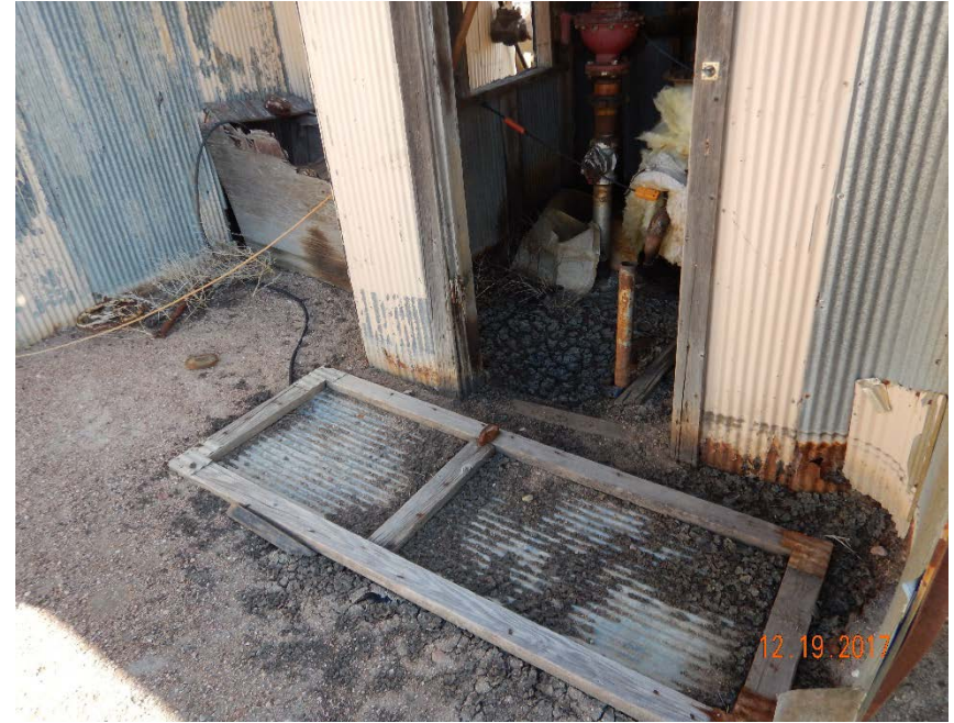
Photo #14 – Junk, debris, stained soil, and unmarked/uncapped flowline riser at entrance to south VHT remain unaddressed from previous FIR. Note that strong hydrocarbon odor and audible gas leak were observed on inspection date.
