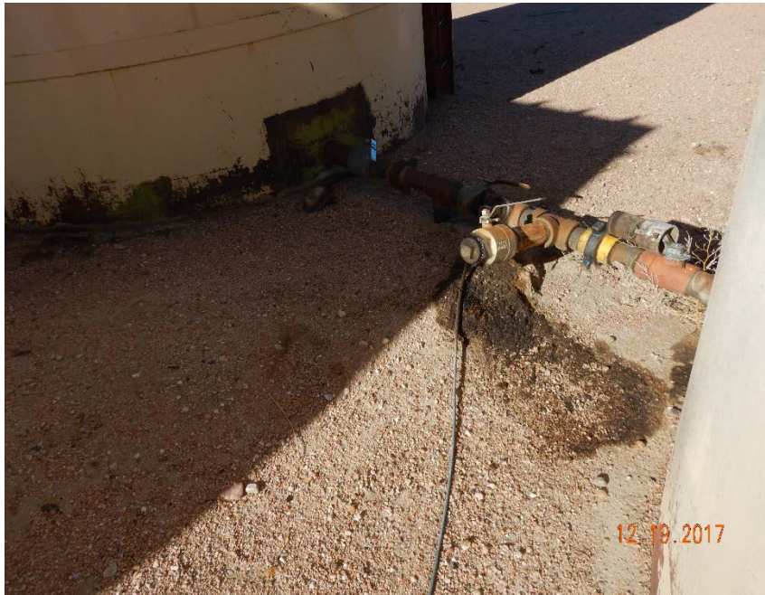
Photo #25 - Localized accumulations of oily waste beneath produced water ASTs and associated equipment (2).
