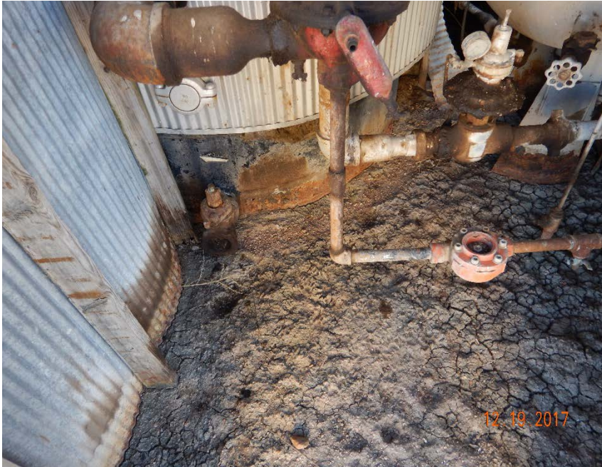
Photo #19 – Oil-stained soil and strong hydrocarbon odor were observed inside of north VHT shed on inspection date.
