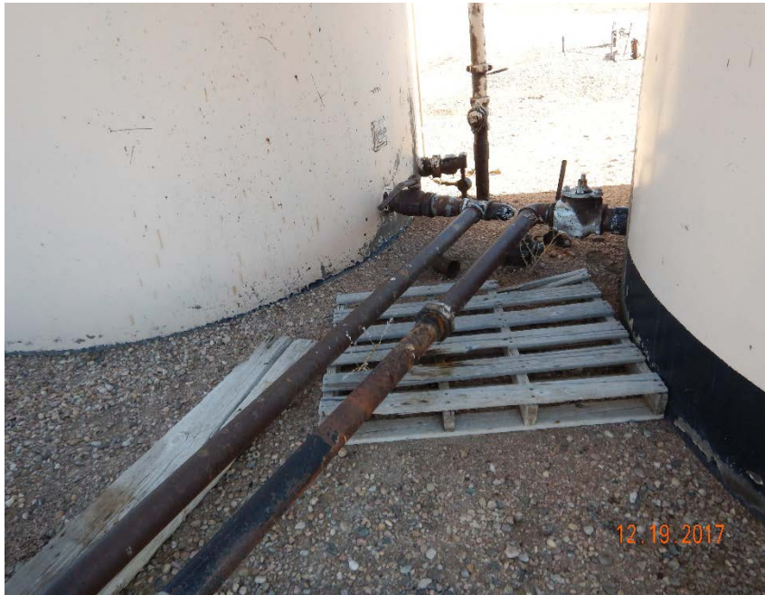
Photo #3 – Wood debris remaining at crude oil ASTs.
