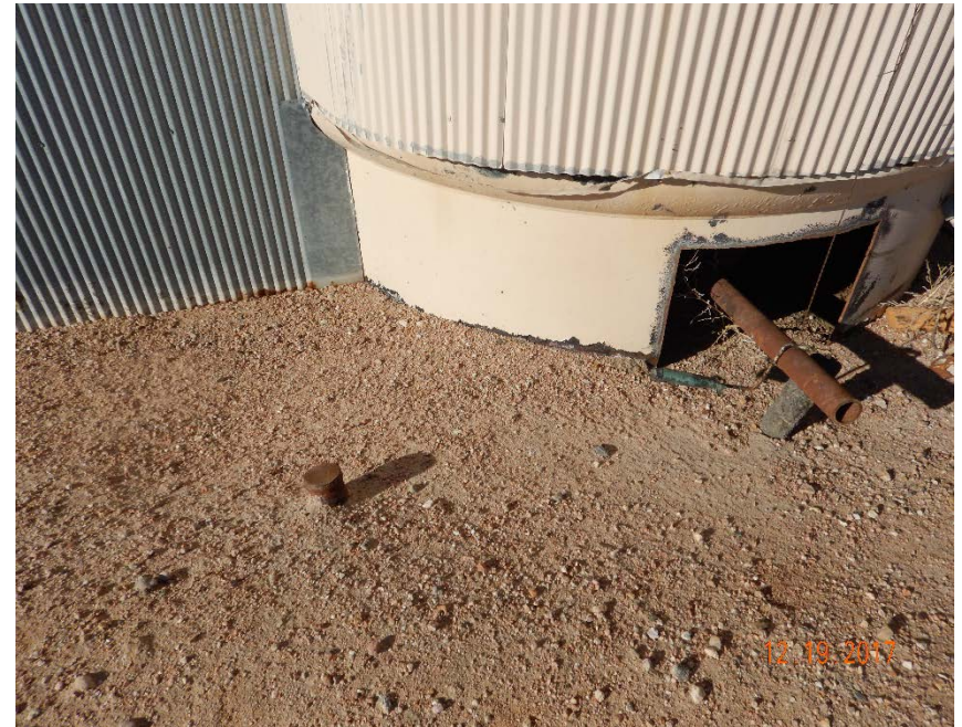
Photo #16 – Capped flowline riser observed on east side of south VHT shed, as indicated in previous FIRs.
