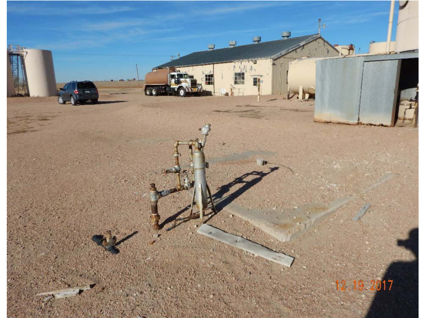
Photo #10 – Unused flowline manifold with concrete slab and wood debris located at SE corner of facility.
