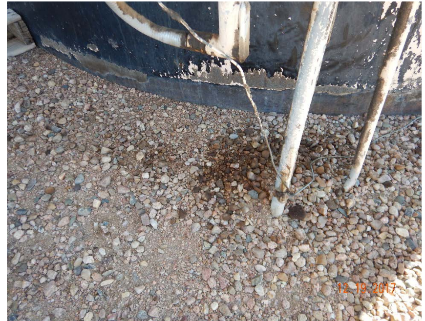
Photo #4 – Localized accumulations of oily waste underlying valves and equipment at crude oil tank battery (1).
