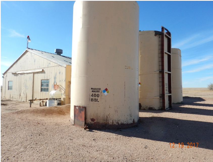
Photo #23 – View of produced water ASTs located north of main building. Note shallow earthen berm.
