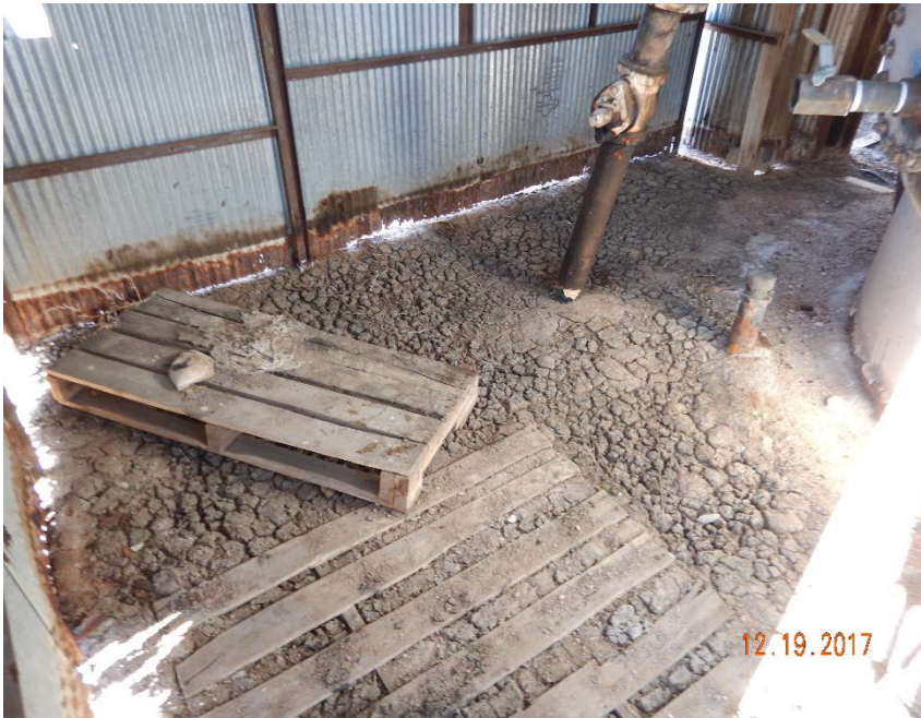
Photo #15 – Oil-stained soil, strong hydrocarbon odor, audible gas leak, and wood debris were observed inside of south VHT shed on inspection date.
