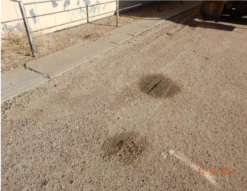
Photo #31 – Localized, oil-stained soil located at SW corner of main building.
