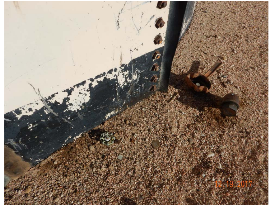
Photo #8 – Flowline riser and valves daylight south of crude oil ASTs.
