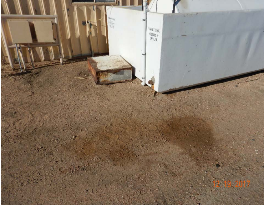
Photo #27 – Localized, oil-stained soil at SE corner of diesel AST.
