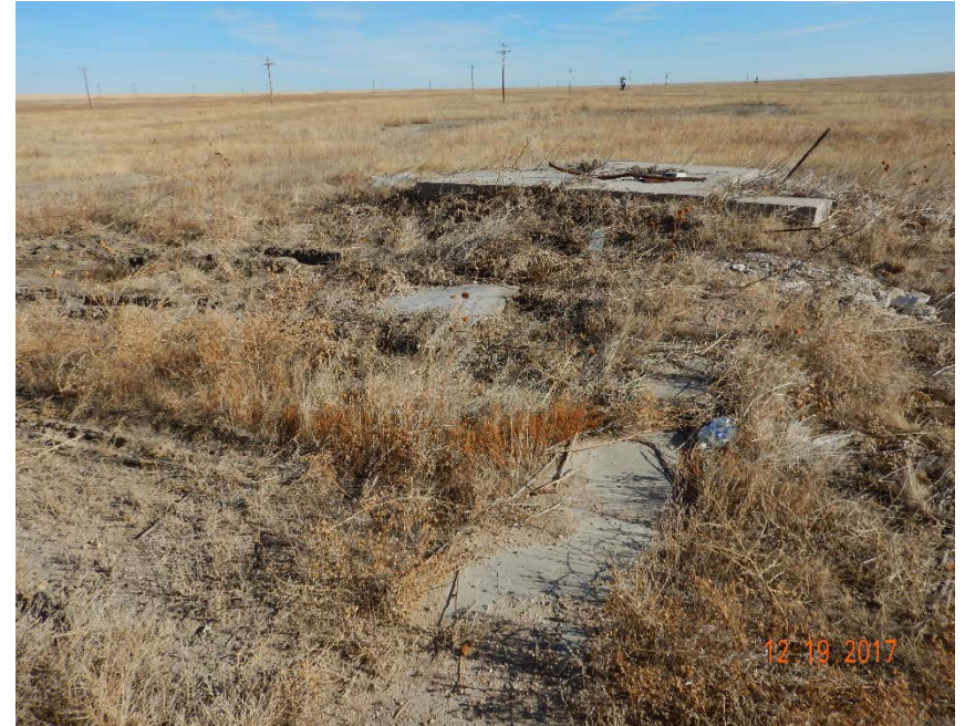
Photo #28 – Unidentified concrete pad with weeds and debris located ~50' east of smaller building on location.
