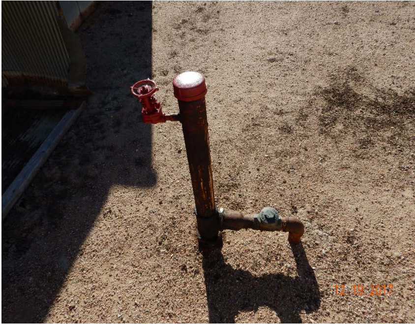
Photo #13 – Flowline risers south of horizontal crude oil AST have been marked by operator in response to previous FIR.
