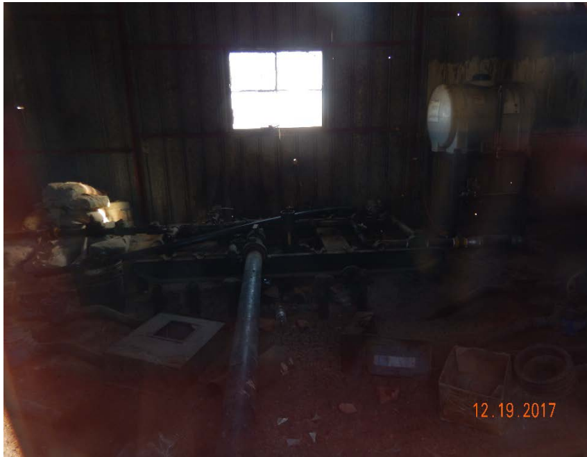
Photo #29 – View inside of small, east building located on east side of facility. See field inspection report #681700672 for additional photos and COGCC instruction to operator to file Form 27 for remediation of environmental impacts.
