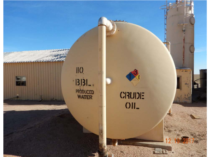
Photo #12 – NFPA placard affixed to west side of horizontal crude oil AST in need of replacement.
