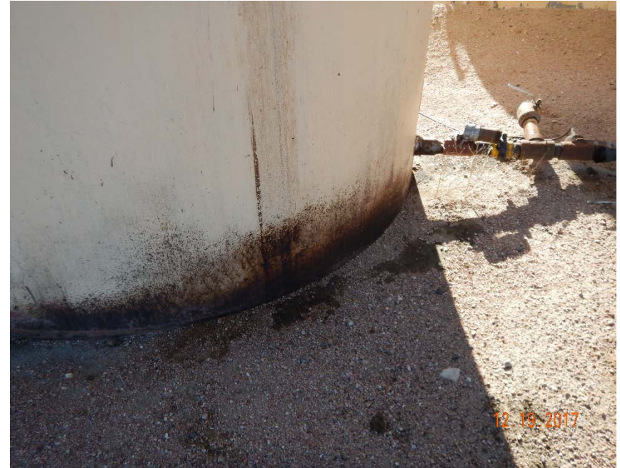
Photo #24 – Localized accumulations of oily waste beneath produced water ASTs and associated equipment (1).
