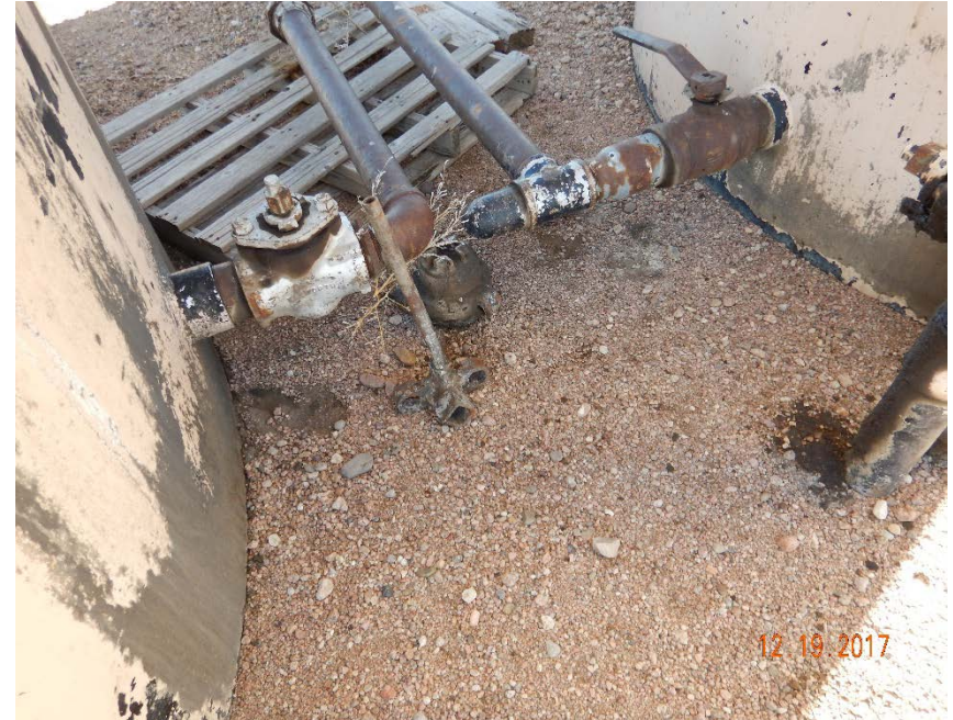
Photo #6 - Localized accumulations of oily waste underlying valves and equipment at crude oil tank battery (3).
