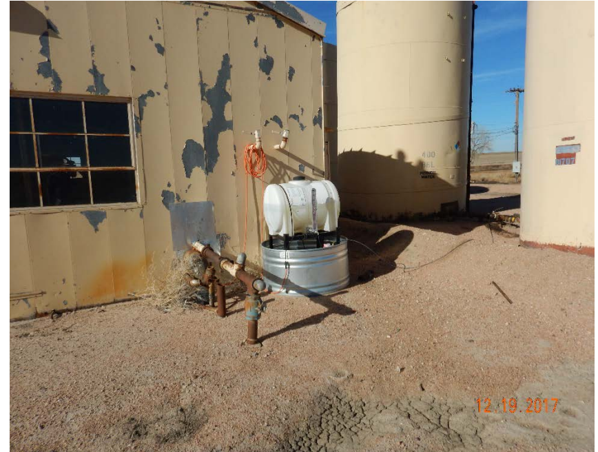
Photo #22 – View of chemical storage tank with metal berm and unused flowline risers at NE corner of main building. Note shallow earthen berm surrounding produced water ASTs.
