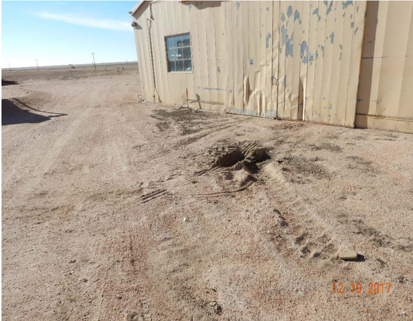
Photo #21 - View of rutted area on east side of main building.
