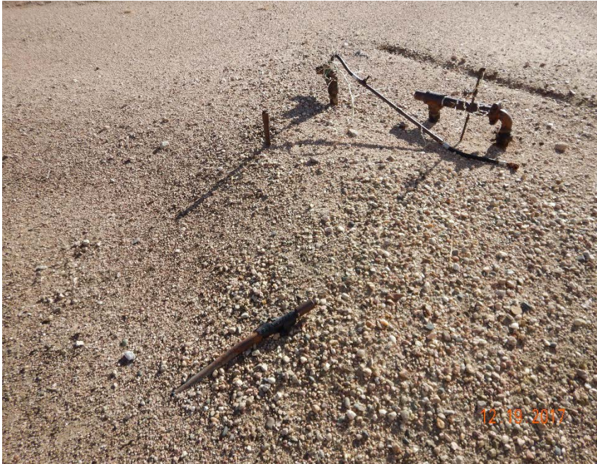
Photo #9 – Unmarked, unused flowline risers daylight east of crude oil ASTs.
