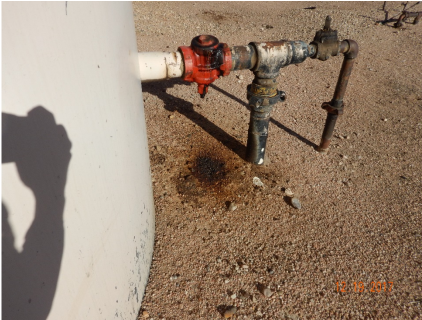
Photo #5 - Localized accumulations of oily waste underlying valves and equipment at crude oil tank battery (2). Note red valve was observed to be actively leaking on inspection date.
