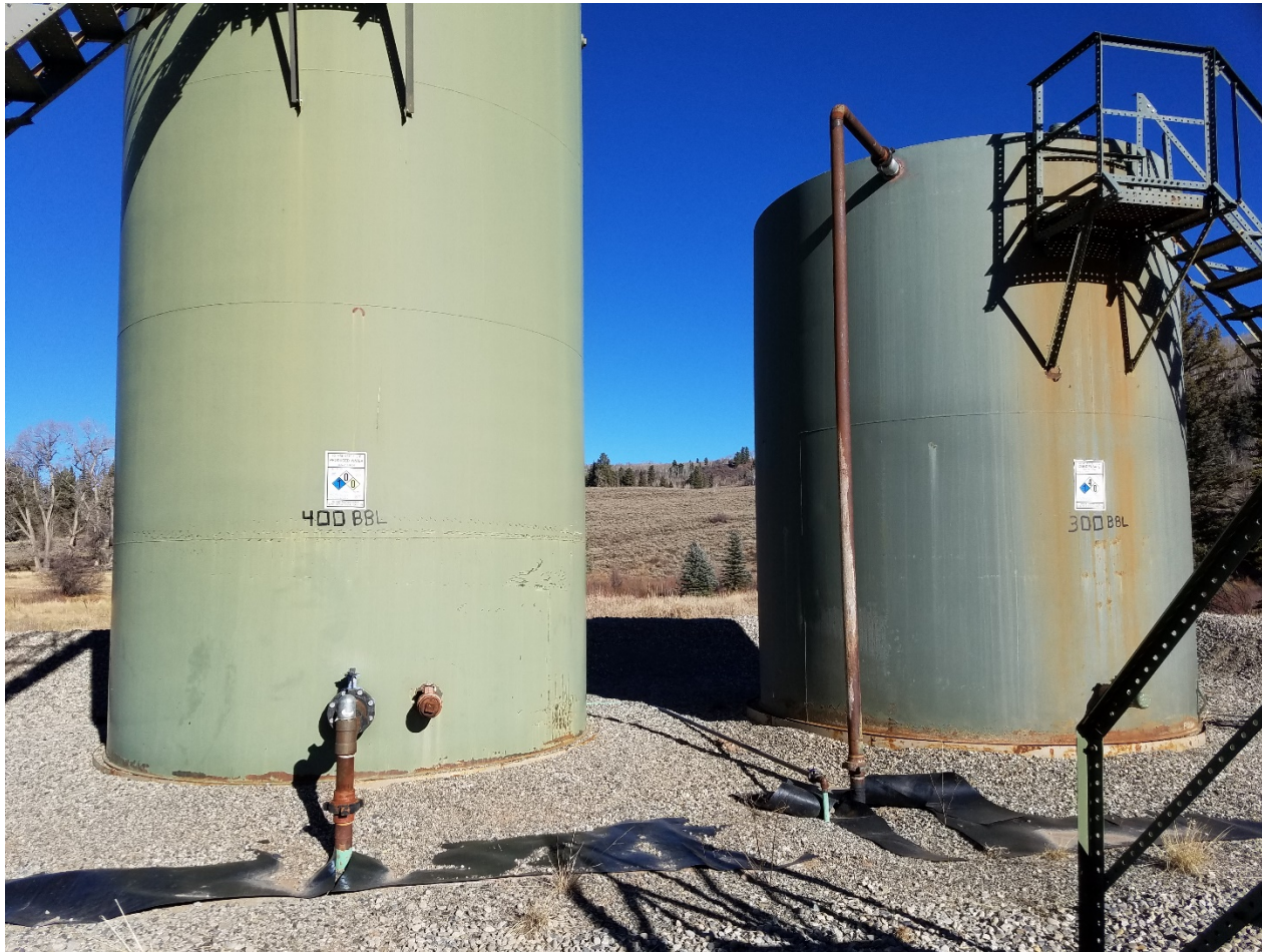
Photo 1. Capacity has been added to tanks. New NFPA labels have been ordered.
