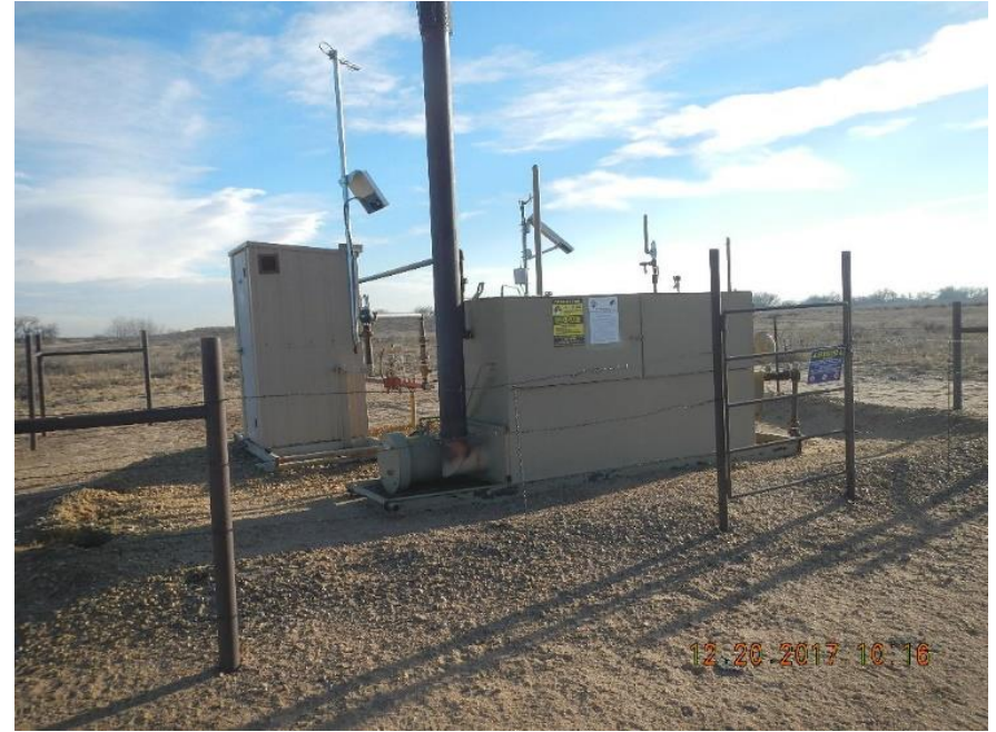
Photo 4 Separator and Gas Meter Run from west
