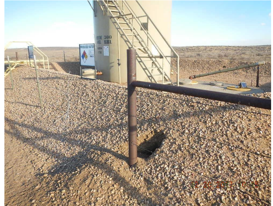
Photo 2 Hole in Berm at Tank Battery from southwest
