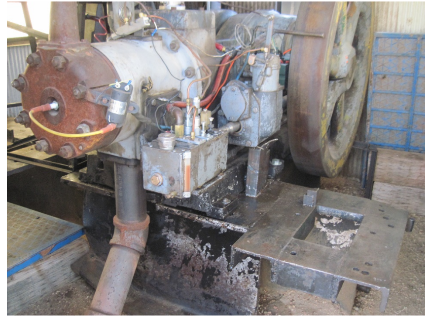
Soiled dirt cleaned up inside pump jack house
