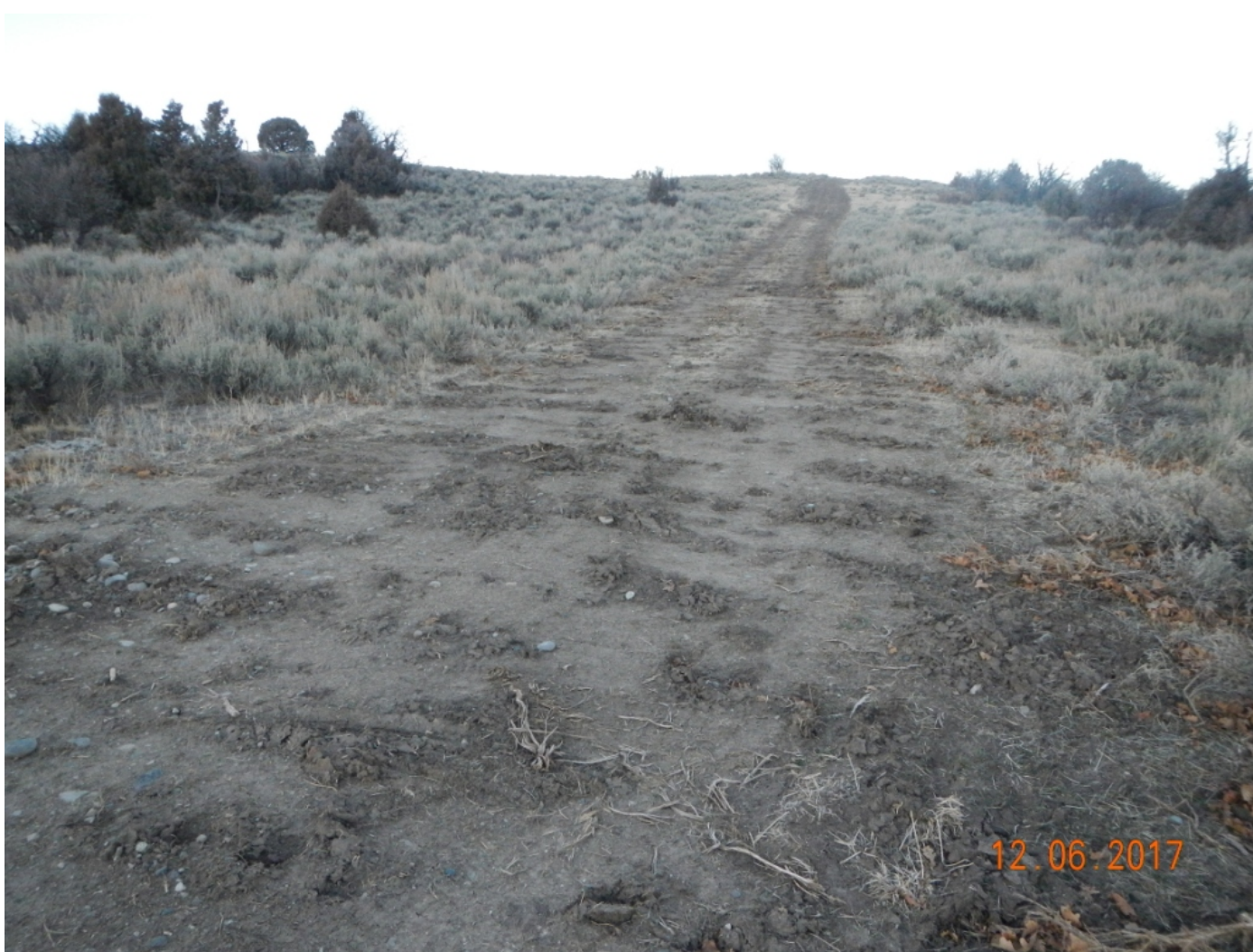
Photo 4. View of area of exposed soils from the access road facing upslope along the pipeline alignment toward the riser at the top of the hill. This area should be seeded and carefully monitored until stabilized.
