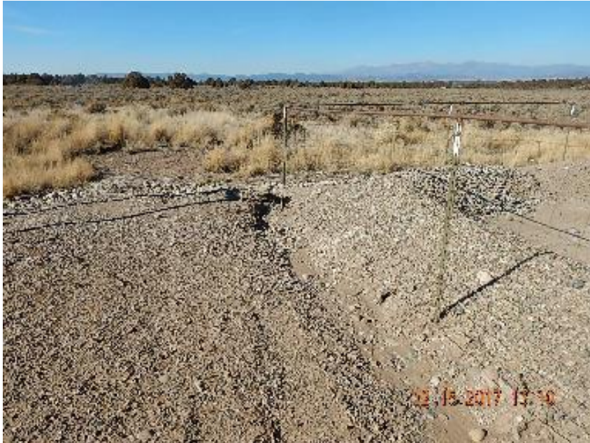
Photo 5: Erosion channel along tank battery berm.
