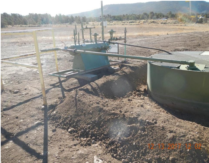
Secondary containment berm maintained to provide adequate capacity.
