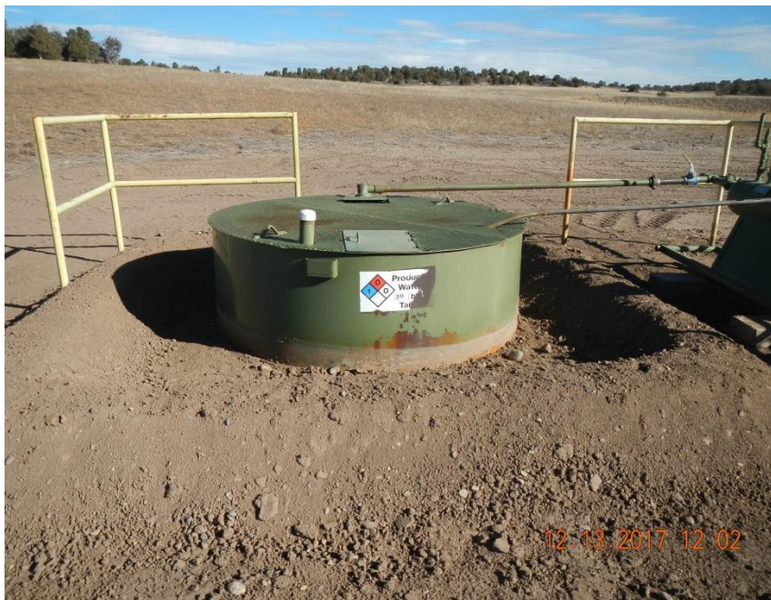
Open topped PW vessel.
