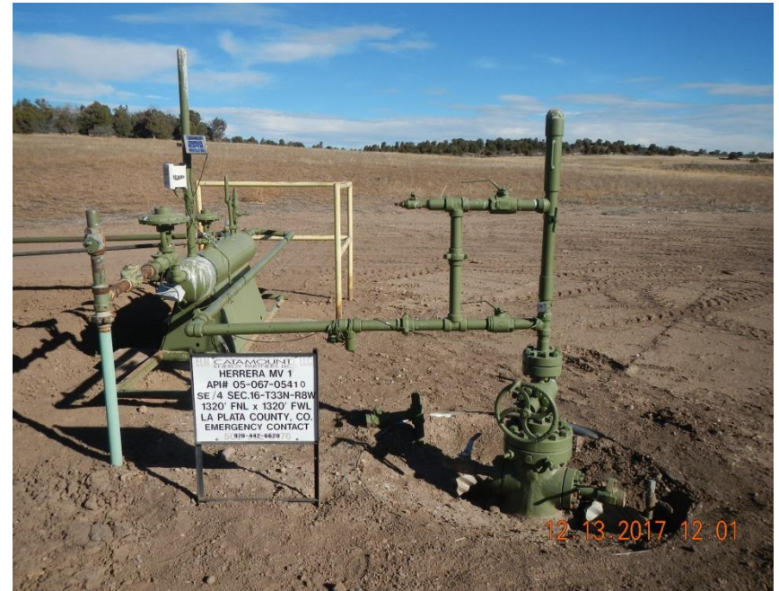
Herrera MV #1 well head and dehy unit.
