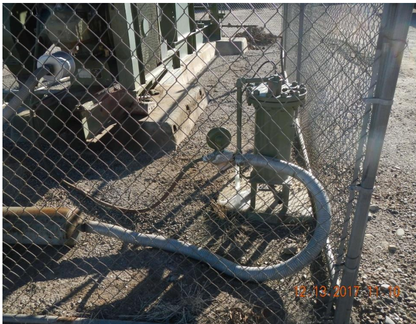
Stained soil noted on inspection document #674901962 has been removed.
