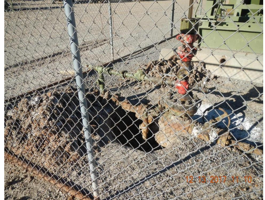
Stained soil and excavation around well head.
