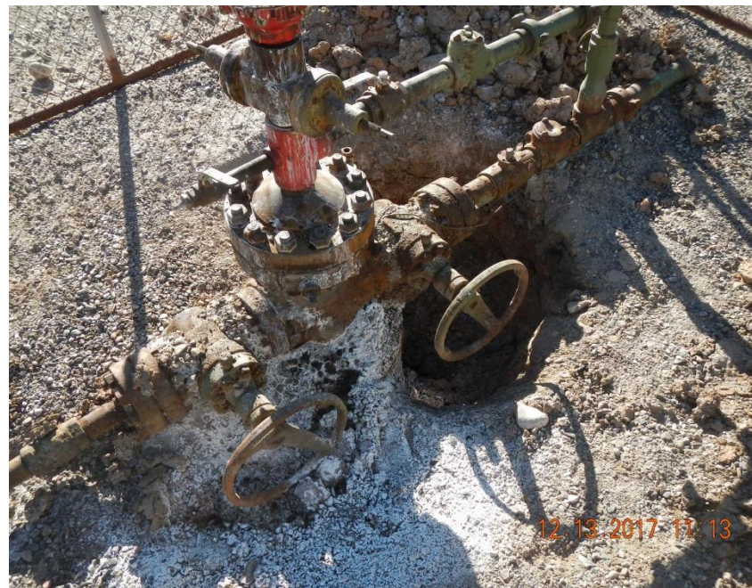
Stained soil and open excavation at well head.
