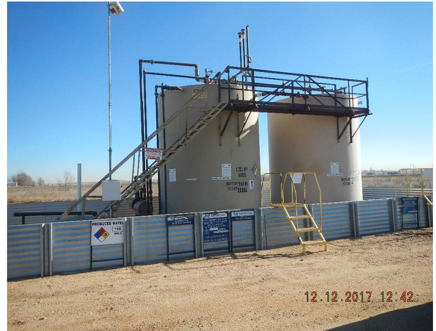
Photo 2 Tank Battery from west
