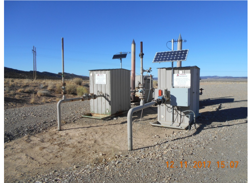
Meter housings and separators with signs
