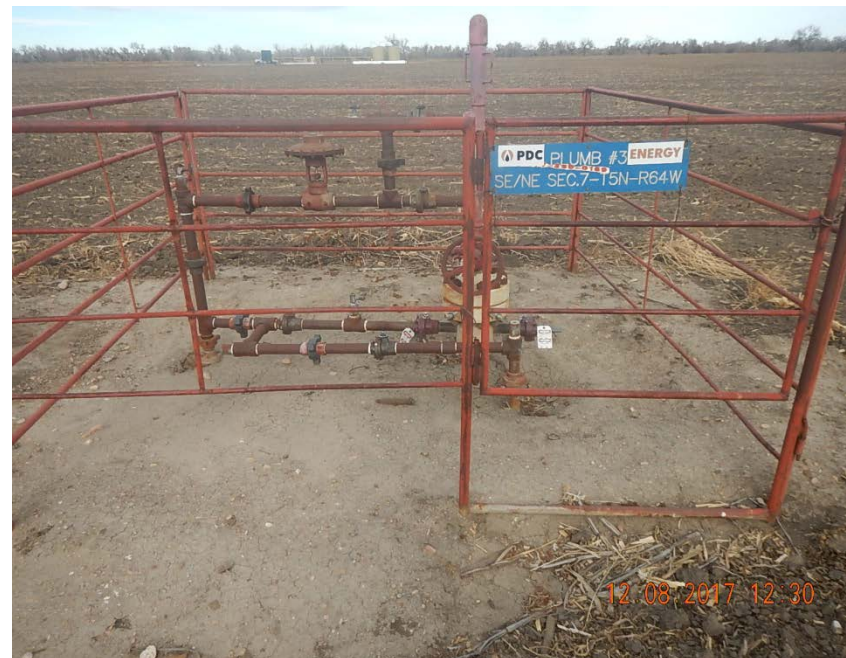
Photo 2: Wellhead, looking N
