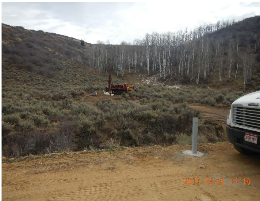
Looking southeast, from the road to A27 CDP. Divide Rd at the top of the ridge. Installing monitoring wells downhill of the Point of Release (POR)
