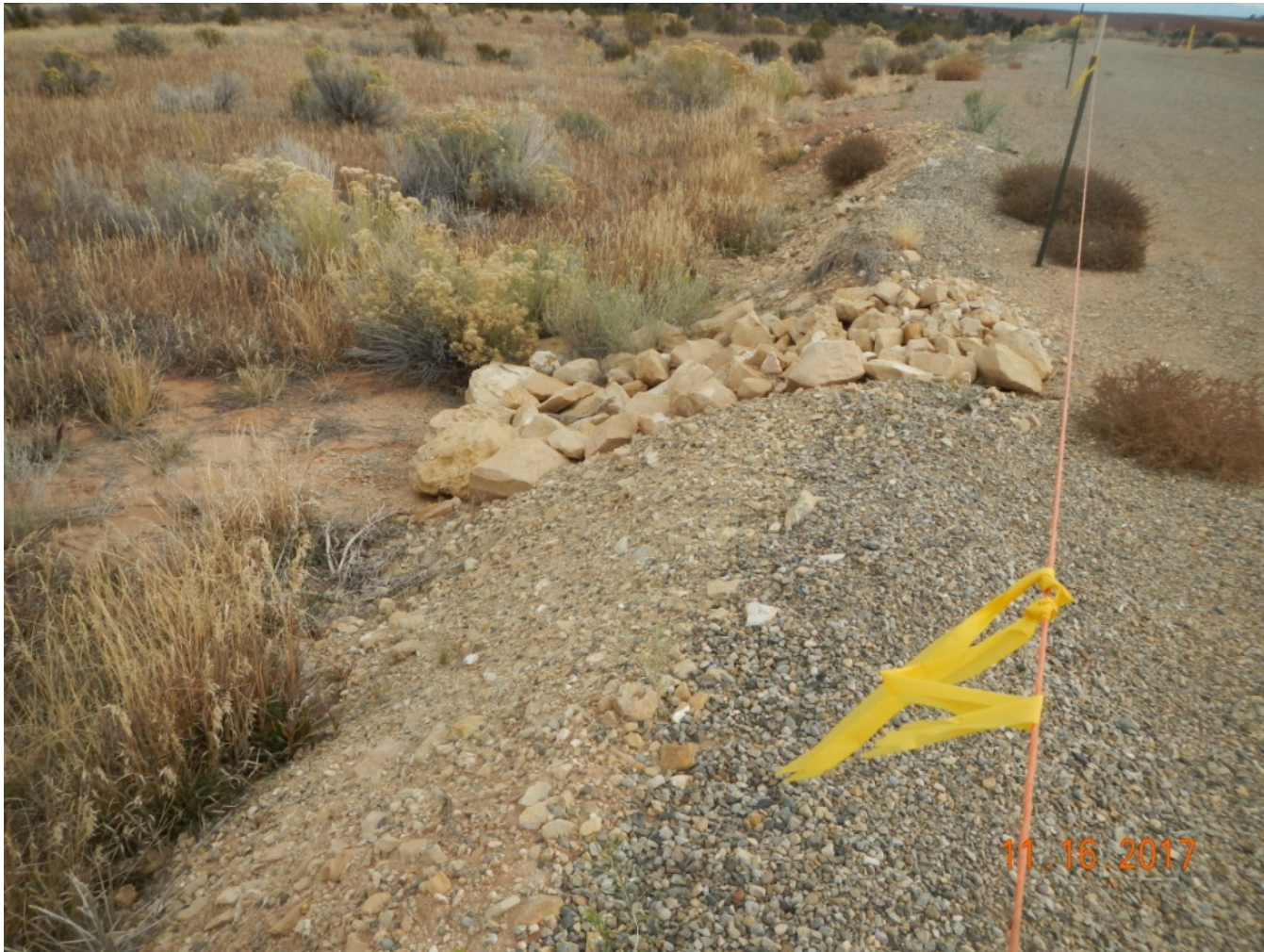
Photo 3. View of rock run-down stormwater controls in the northern portion of the project area.
