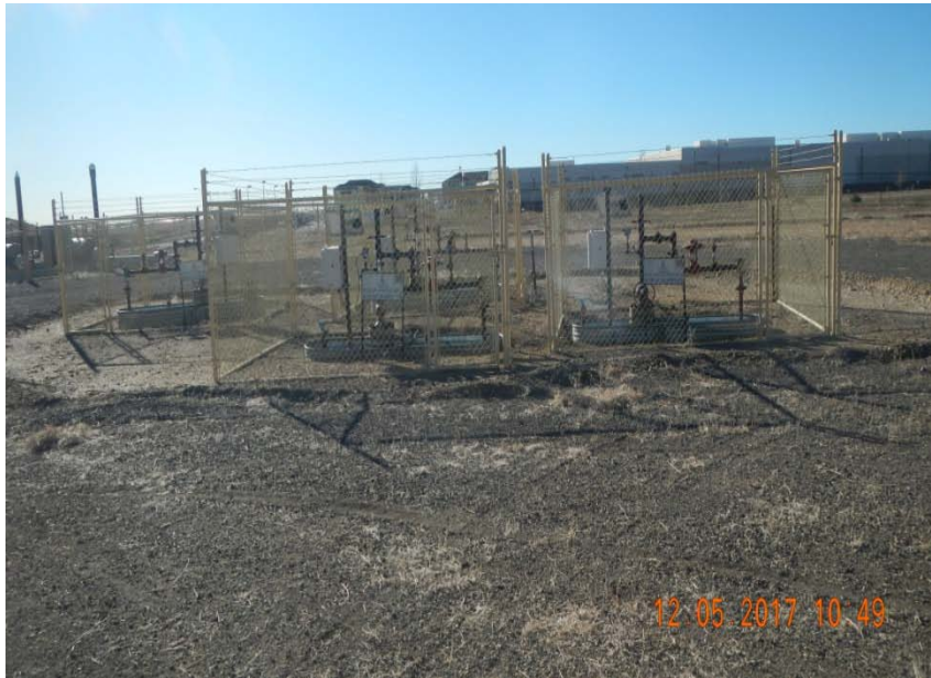
Wells on battery
