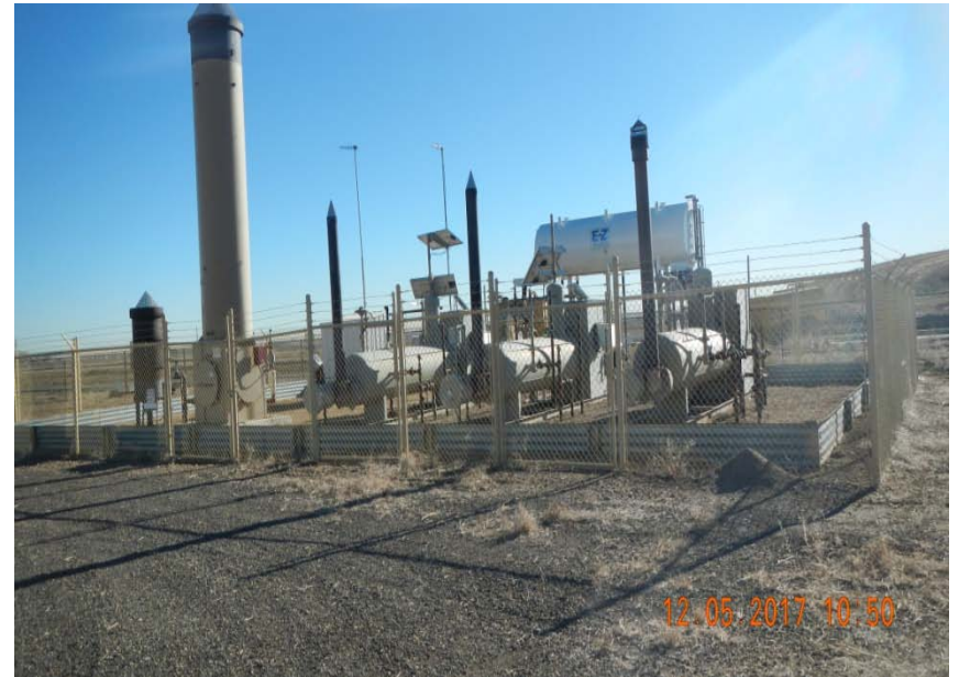
Separators, ECDs, Meter Run.
