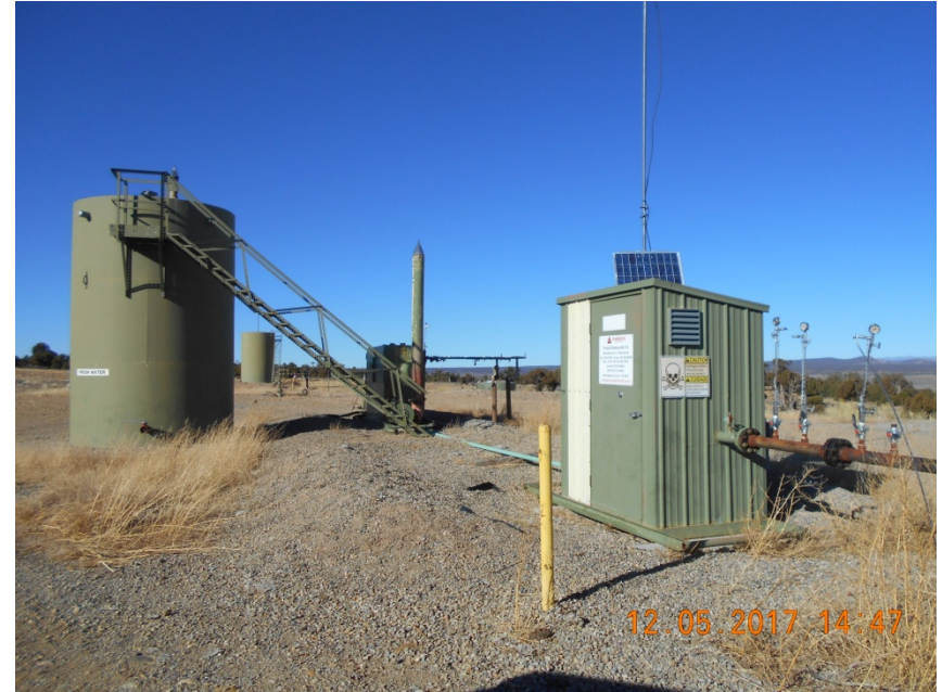
Meter housing with sign, Separator and tanks.
