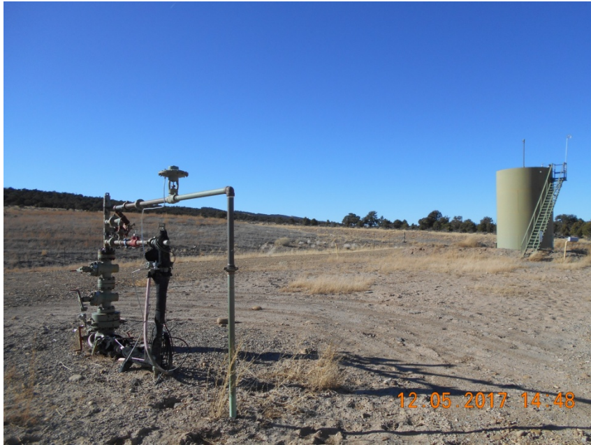
Wellhead and Produced Water tank.
