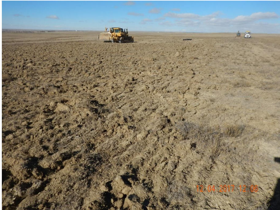
Photo 7: Photo taken from the southeast corner of the location, facing north. Photo shows surface roughening along the perimeter of the location
