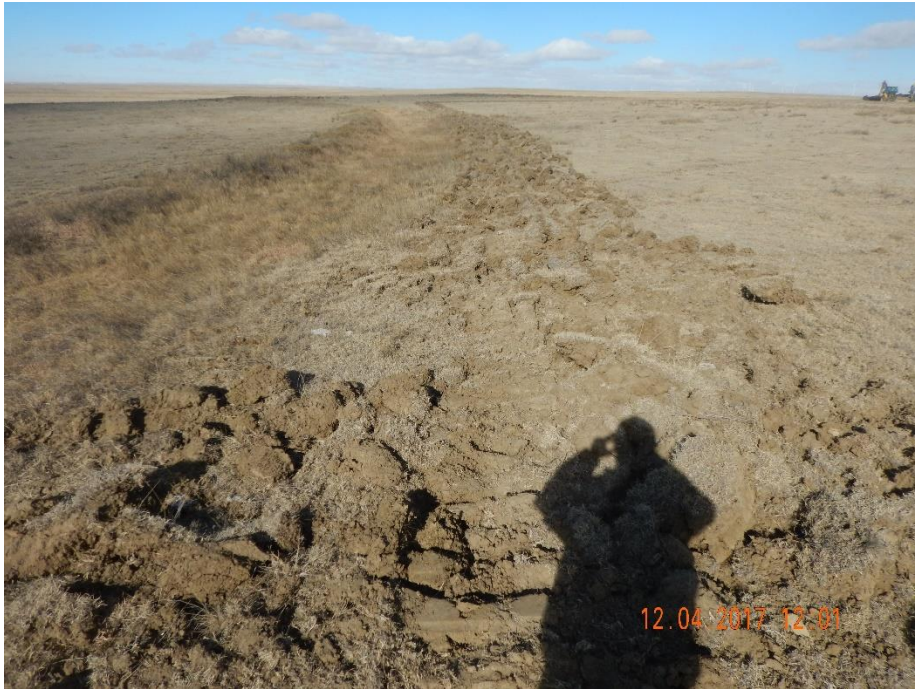
Photo 1: Photo taken from the southwest corner of the location, facing north. Photo shows surface roughening along the perimeter of the location. Photo also shows a pre-existing ditch on the west end of the location that operator has incorporated into the SW BMPS.
