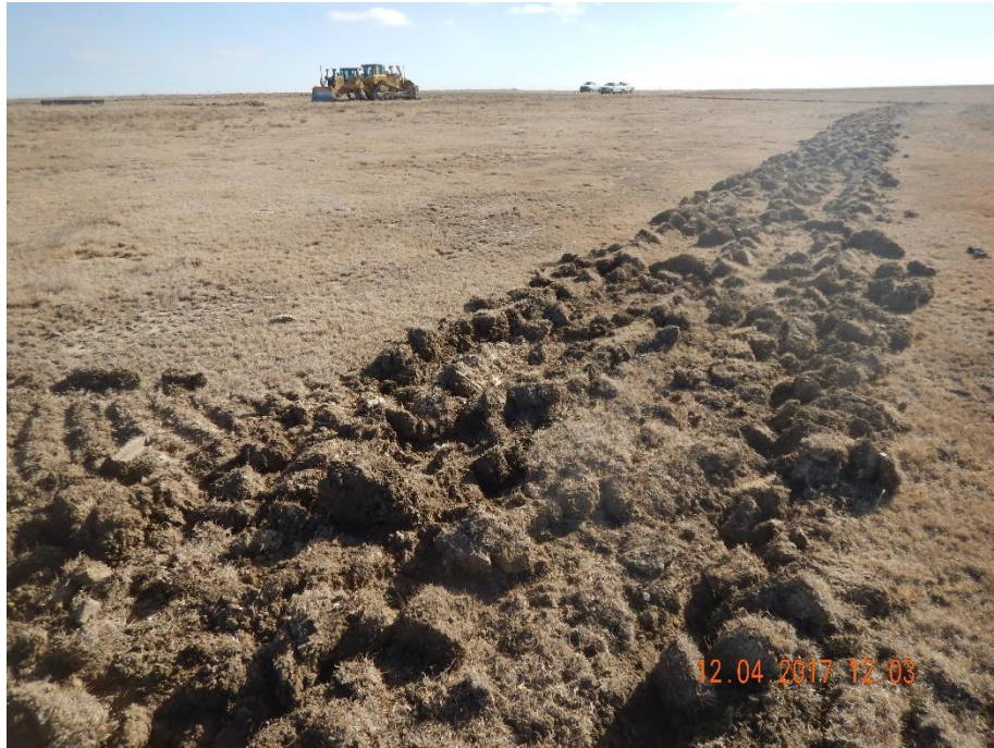
Photo 3: Photo taken from the northwest corner of the location, facing south. Photo shows surface roughening along the perimeter of the location
