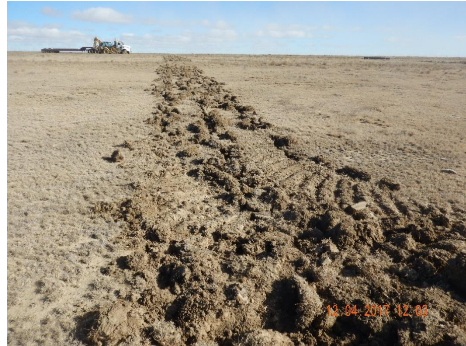
Photo 4: Photo taken from the northwest corner of the location, facing east. Photo shows surface roughening along the perimeter of the location
