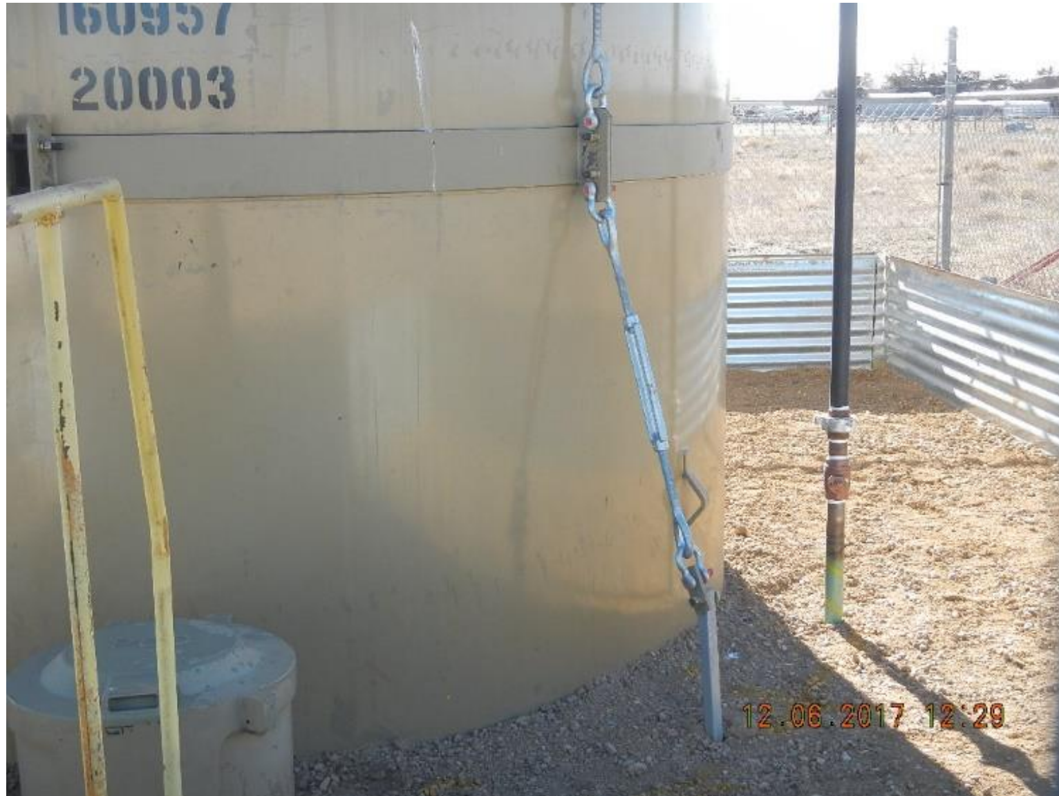
Flood Anchor on Crude Oil Tank
