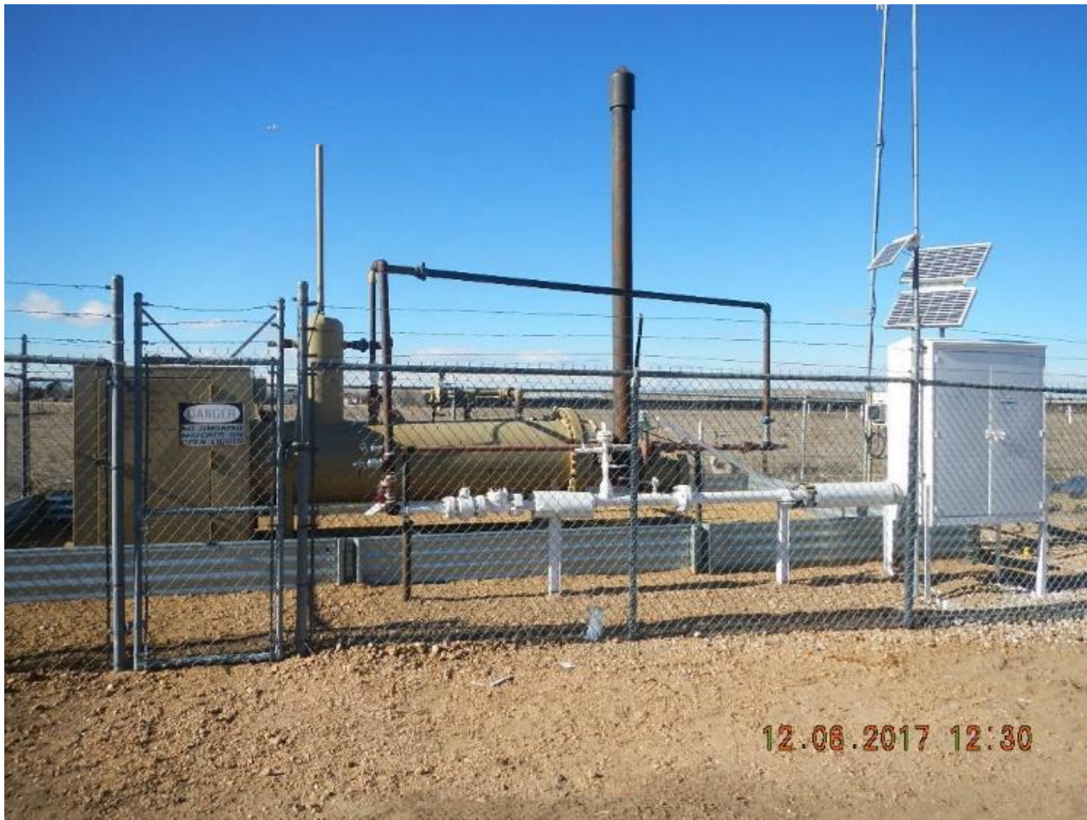
Separator and GMR from east
