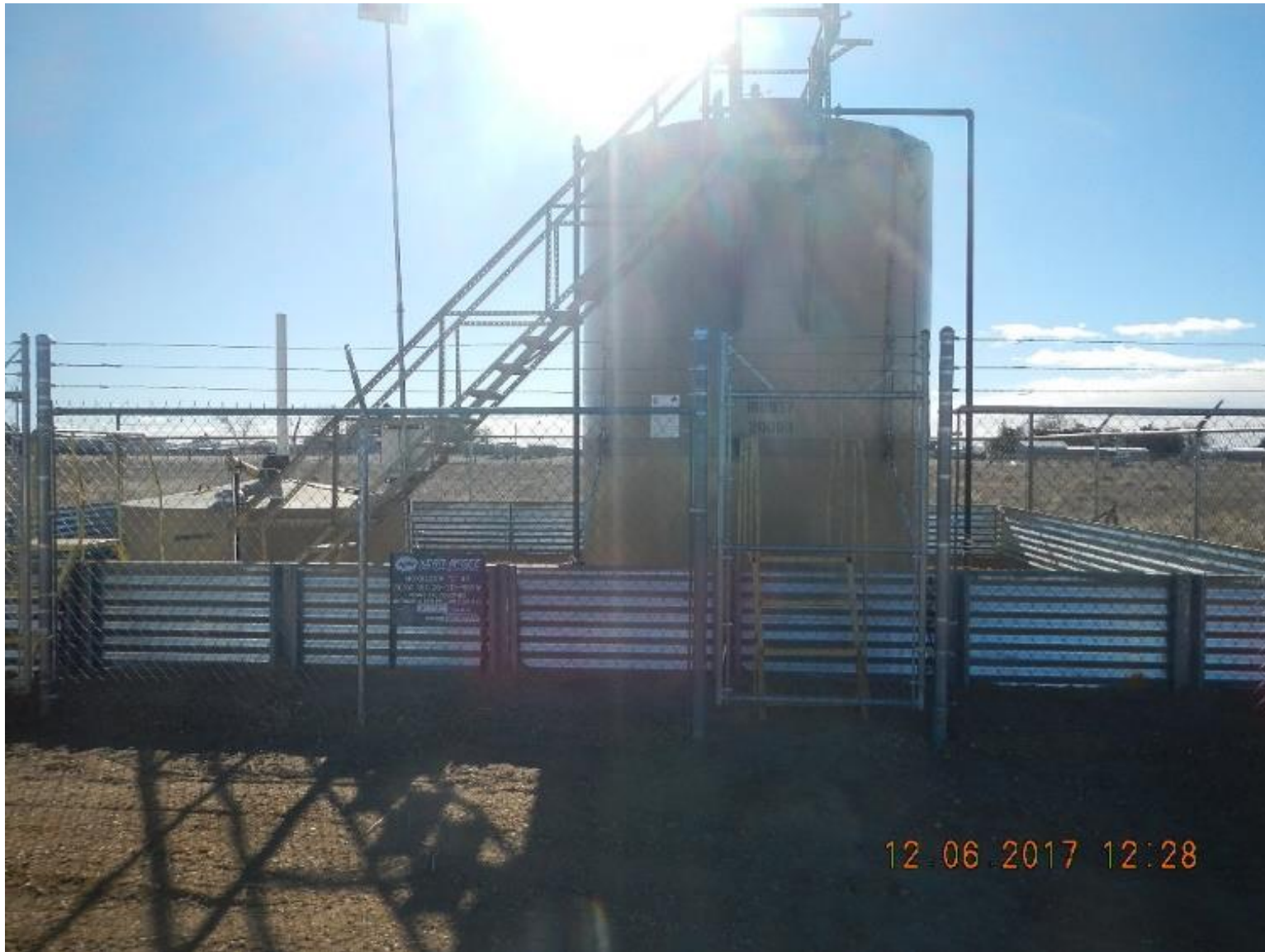
Battery from north Location Number: 319858
