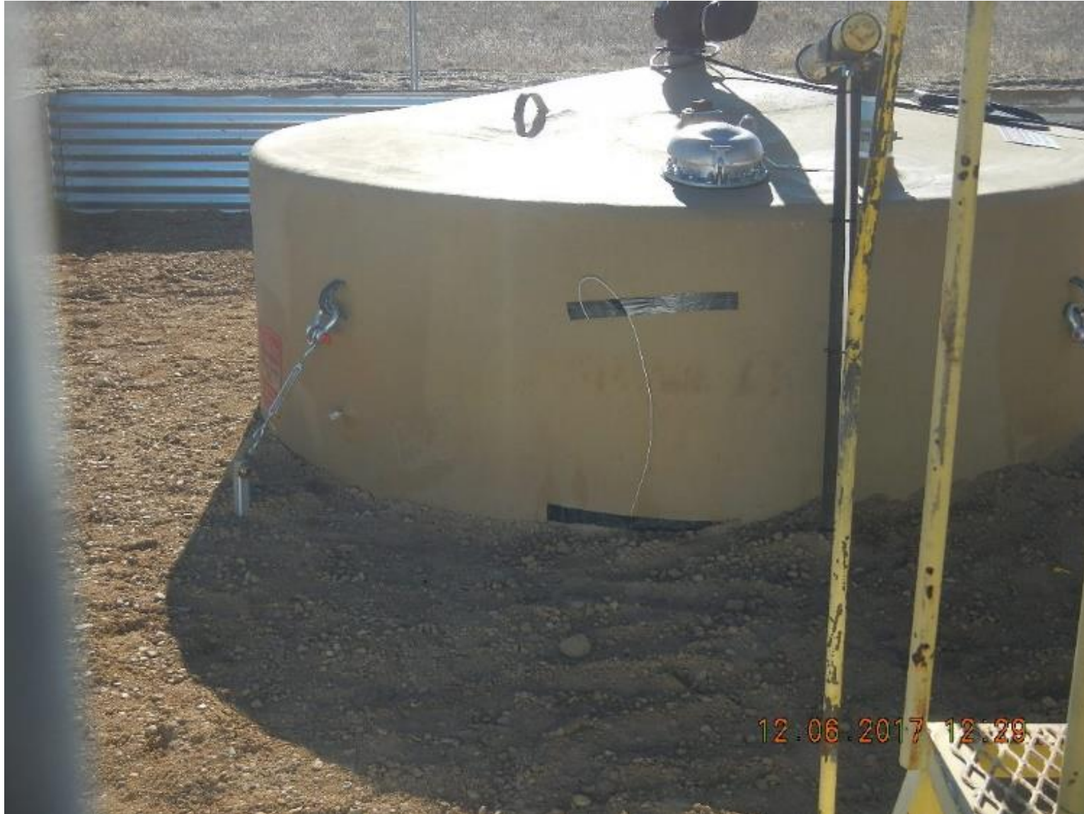
Flood Anchor on Produced Water Tank Location Number: 319858
