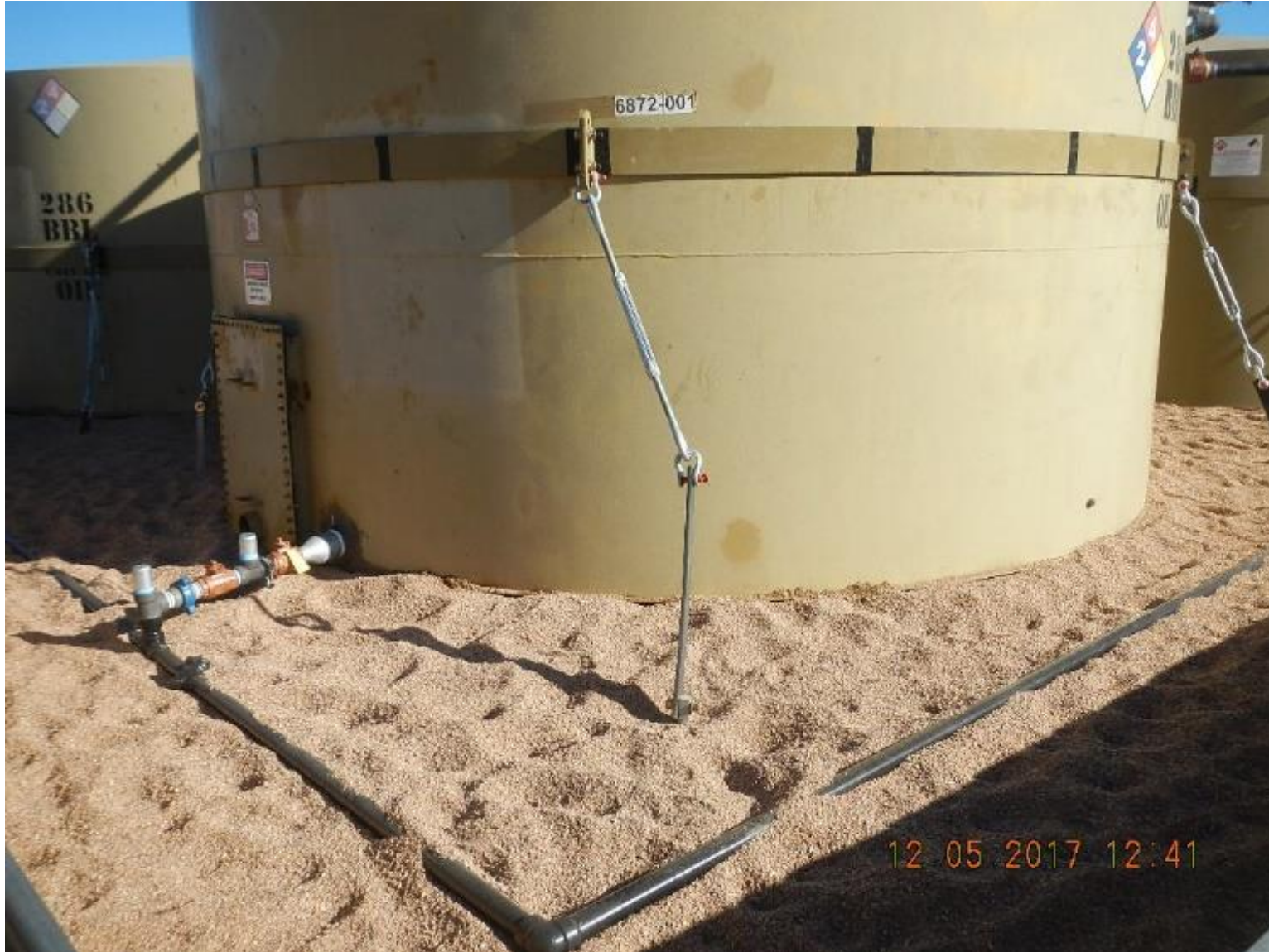
Crude Oil Tank Flood Anchoring Location Number: 333268
