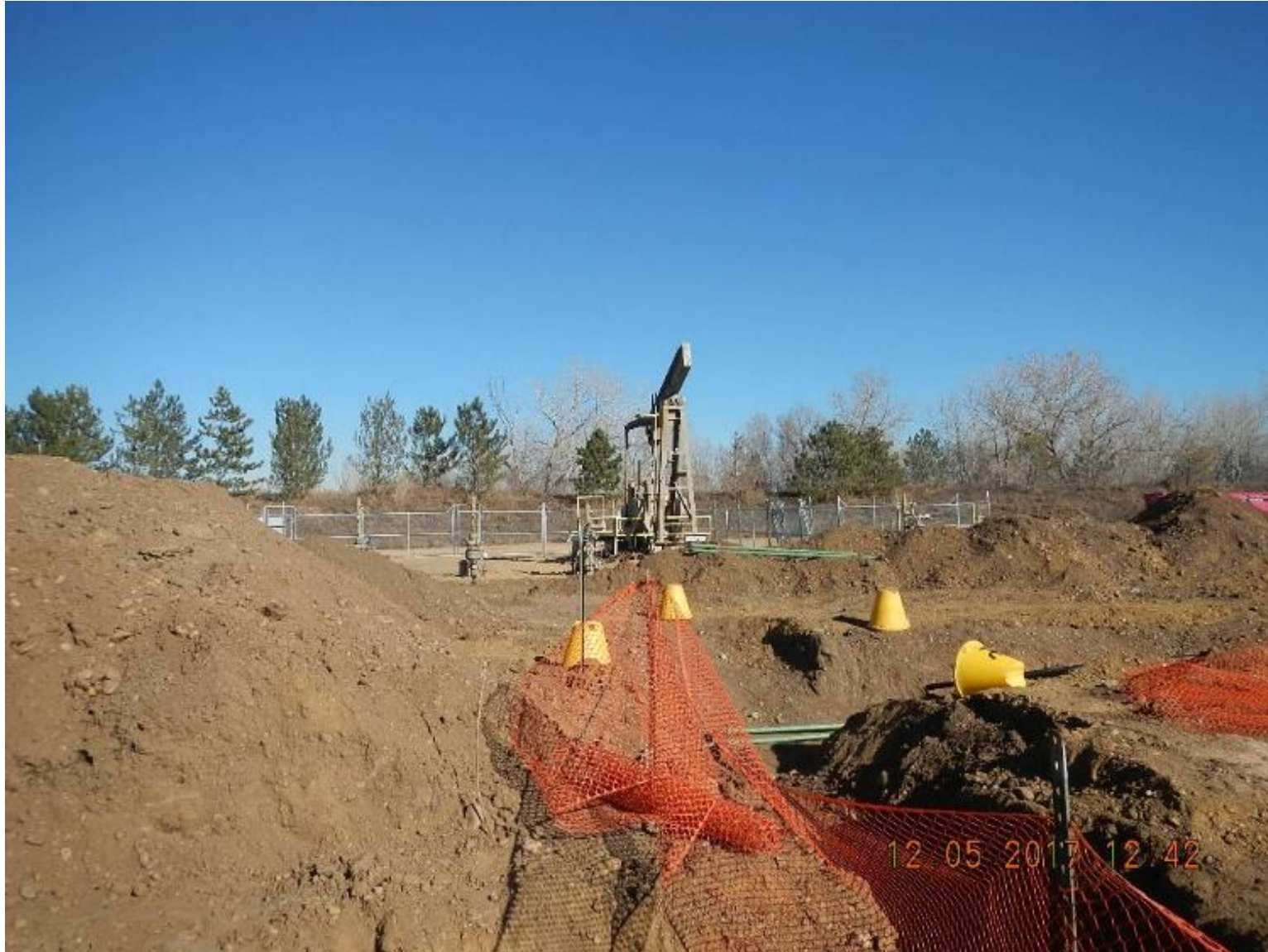
Wellheads from South Location Number: 333268
