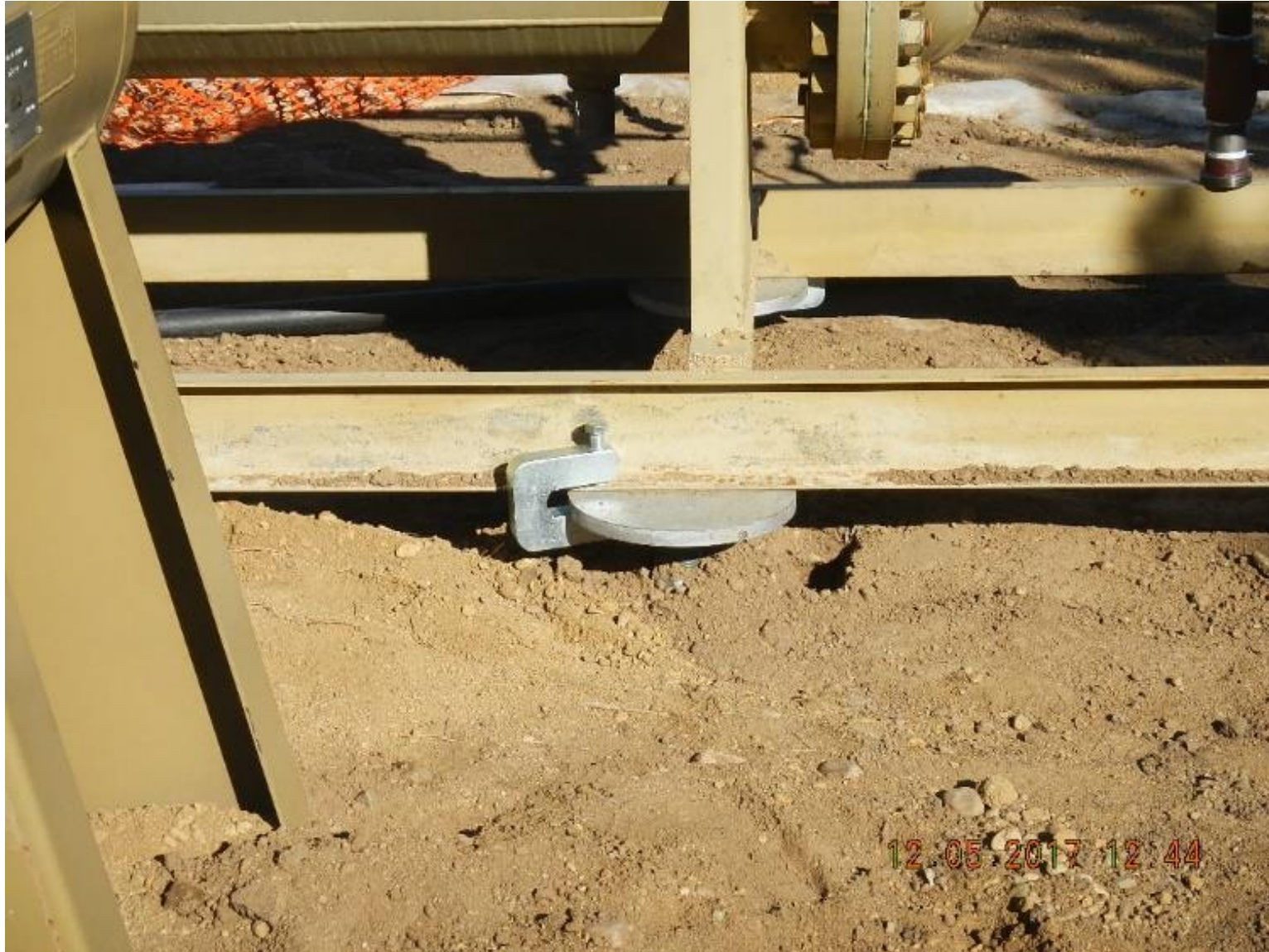
Separator Flood Anchoring Location Number: 333268
