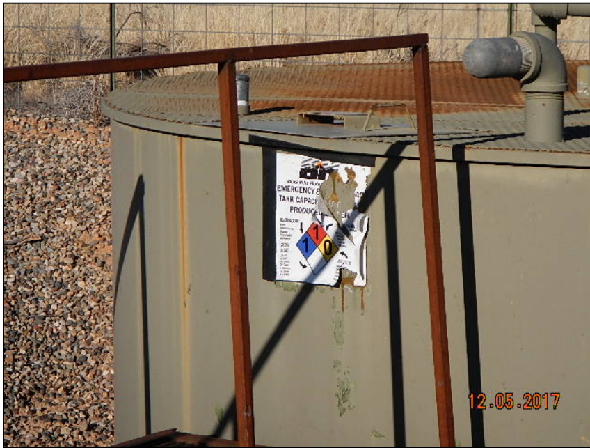
Photo 1. Tank sign is peeling and parts are illegible.
