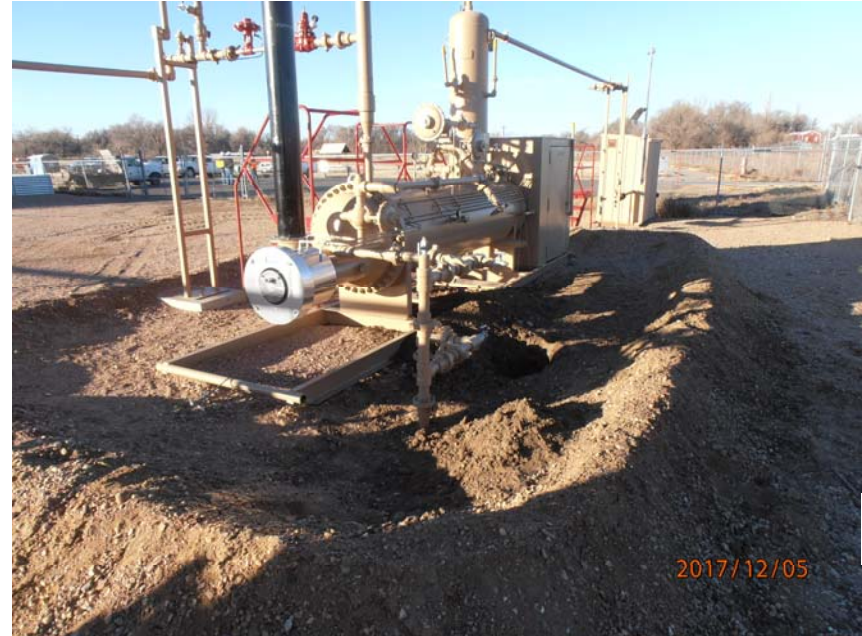
Photo 4 – Separator at Bunn M 1-34 production facility.
