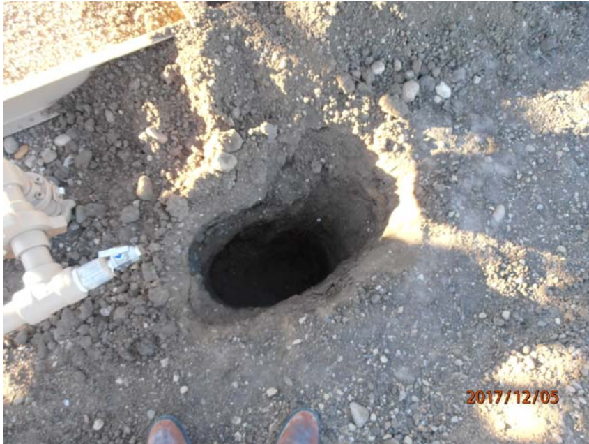
Photo 3 – Pothole at separator at former location of the abandoned McIntyre 34-16 flowline riser.
