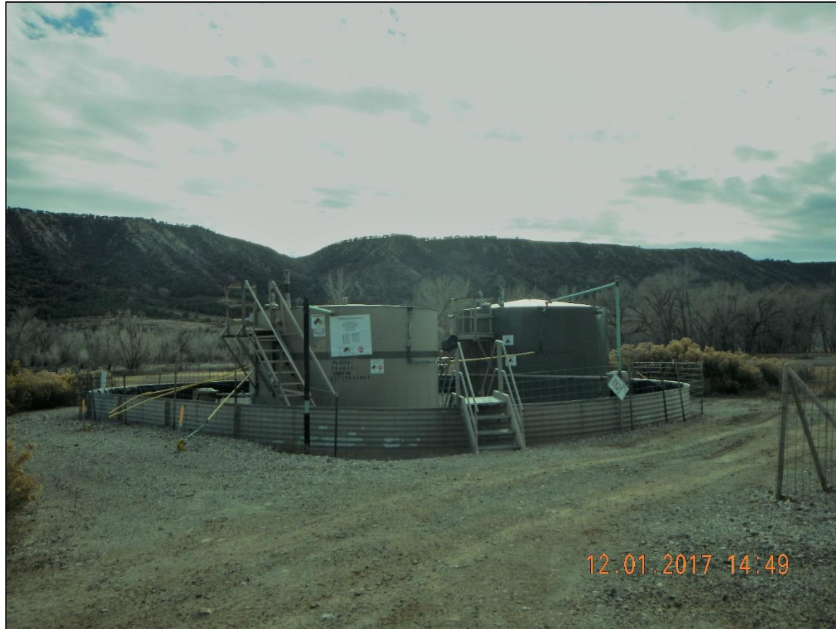
North view of tanks. Tanks anchored with cables and ground anchors.
