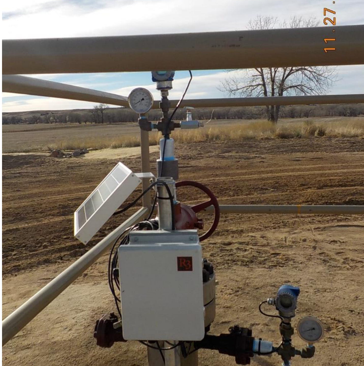
Wellhead pressure monitoring equipment
