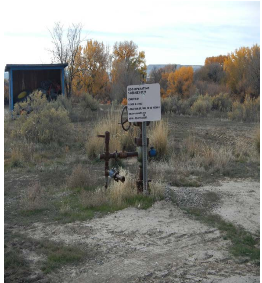
Photo#2: View South over Location Center Note debris weeds within 25Ft of Well Head area.
