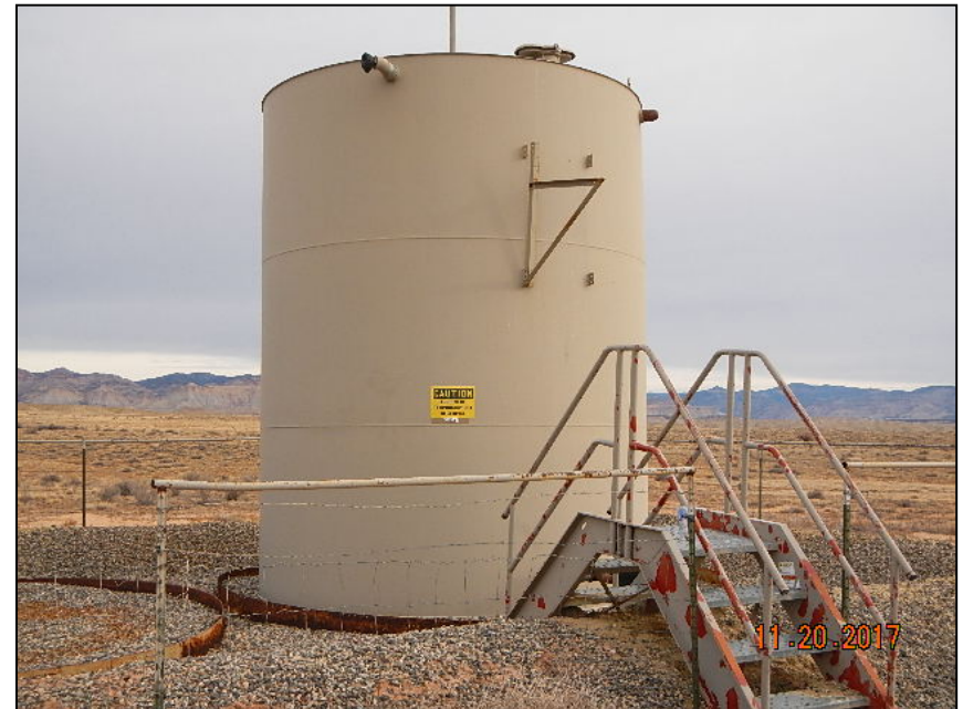
Photo 2. Out of service tank.
