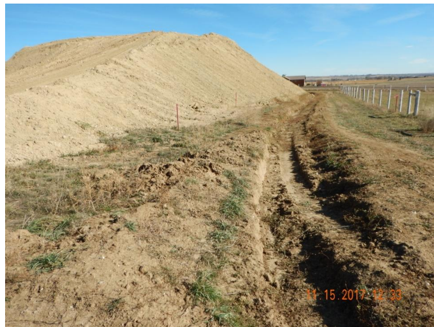
Photo 2. Photo taken from the southeastern location, facing East. Ditch BMP installed around the perimeter of the location. Ditch depth appeared shallow along portions. Stockpile has been constructed to a significant height and may need additional stabilization as rill erosion was observed along portions of the stockpile.
