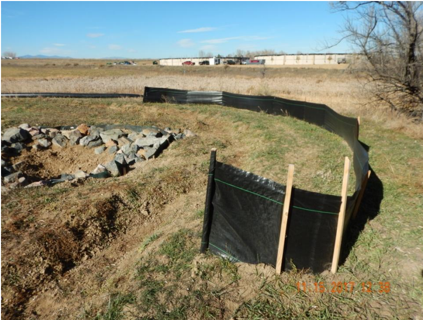
Photo 5. Photo taken from the northern location, facing Northwest. Silt fence BMP constructed around the stabilized outlet area of the sediment basin.
