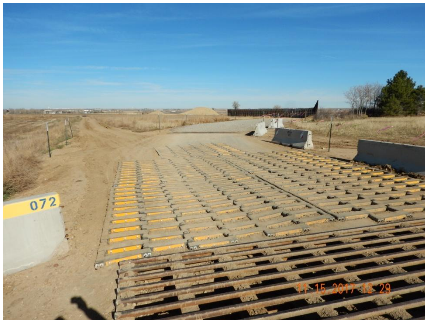
Photo 1. Photo taken from the entrance of location, facing North. Tracking pad devices installed at location.
