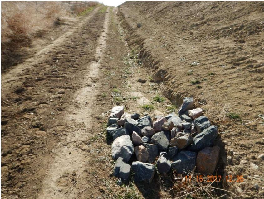
Photo 3. Photo taken from the eastern location, facing South. Check dam BMP installed along portions of the eastern ditch BMP. See comments under Photo 2.
