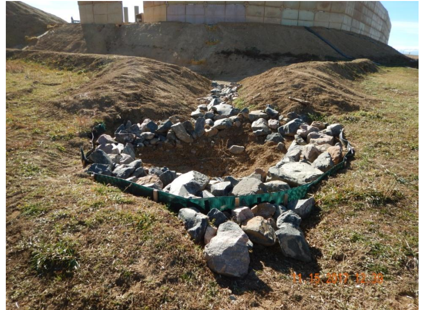
Photo 6. Photo taken from the northern location, facing South. Rip-rap and S-Fence have been installed for the stabilized outlet area.
