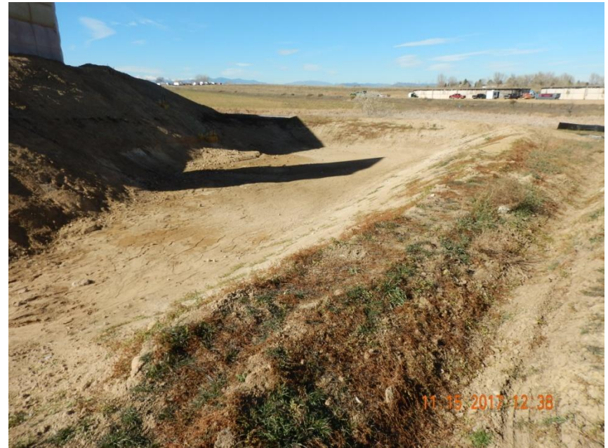
Photo 4. Photo taken from the northern location, facing West. Sediment basin has been installed with a stabilized outlet.
