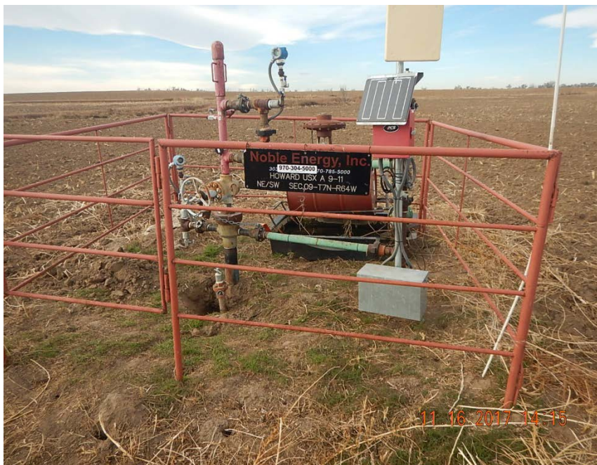
Photo 1: Wellhead, looking NW
