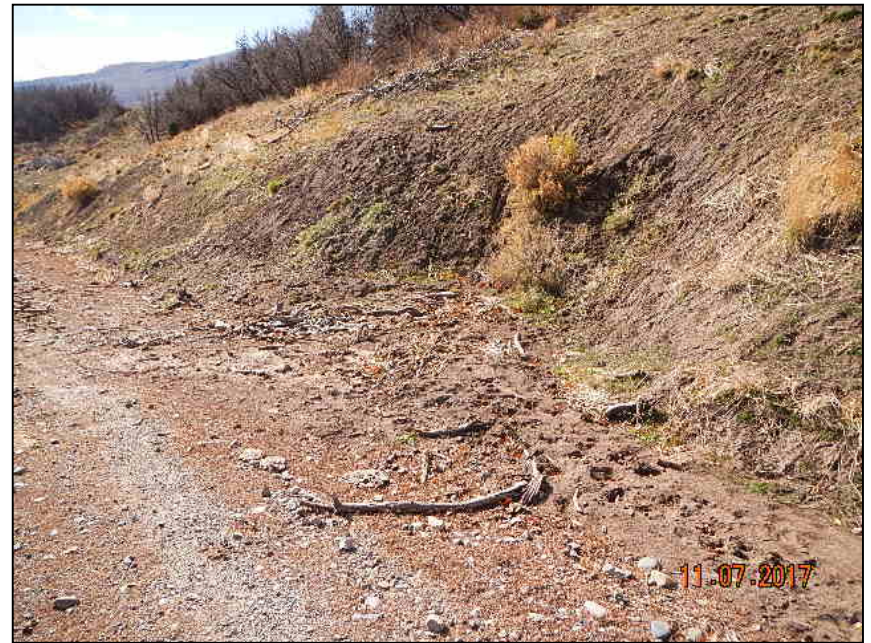
Photo 6. Silted in inlet to culvert
