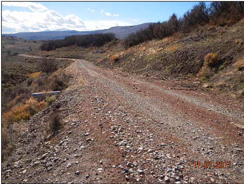
Photo 5. one of two culverts with silted in inlet.
