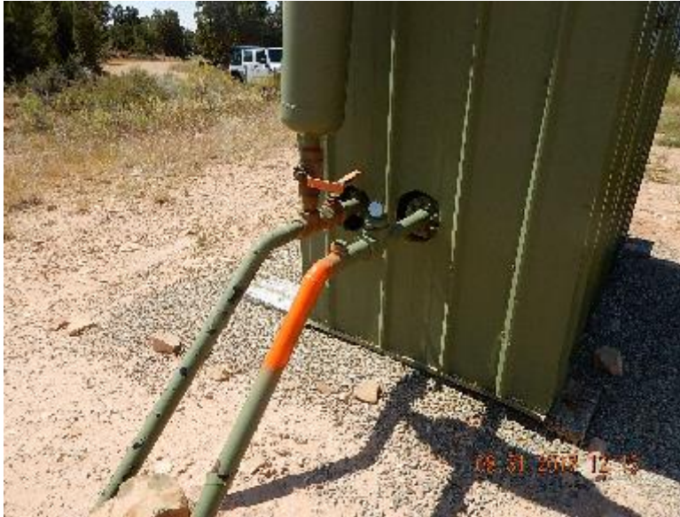
Photo 5: Flowline riser at meter house open to atmosphere. Previous inspection.
