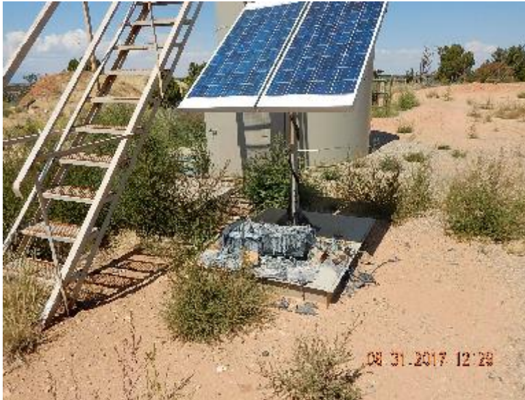
Photo 11: Burnt batteries under solar panel. Previous inspection.
