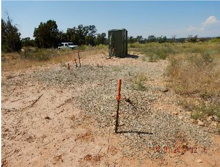
Photo 7: (4) risers off backside of gas meter run shed. Previous inspection.
