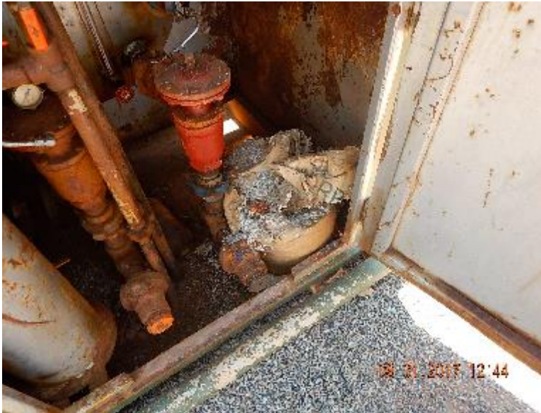
Photo 13: Deteriorated bag of material inside separator box. Previous inspection.
