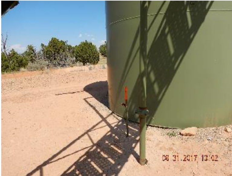
Photo 9: Riser in production tank battery. Previous inspection.
