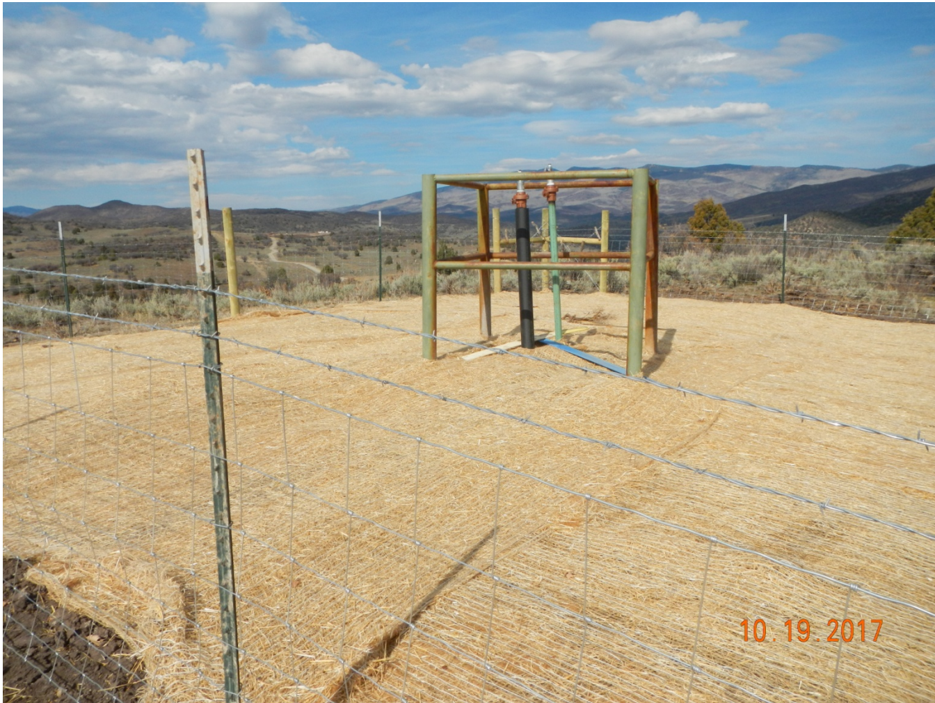
Photo 1. View of area recently reclaimed around pipeline riser. Area is recently reclaimed.
