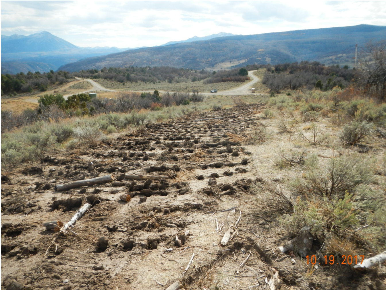
Photo 3. View of area south of repaired riser that was recently reclaimed. Area is surface roughened and appears to be seeded.
