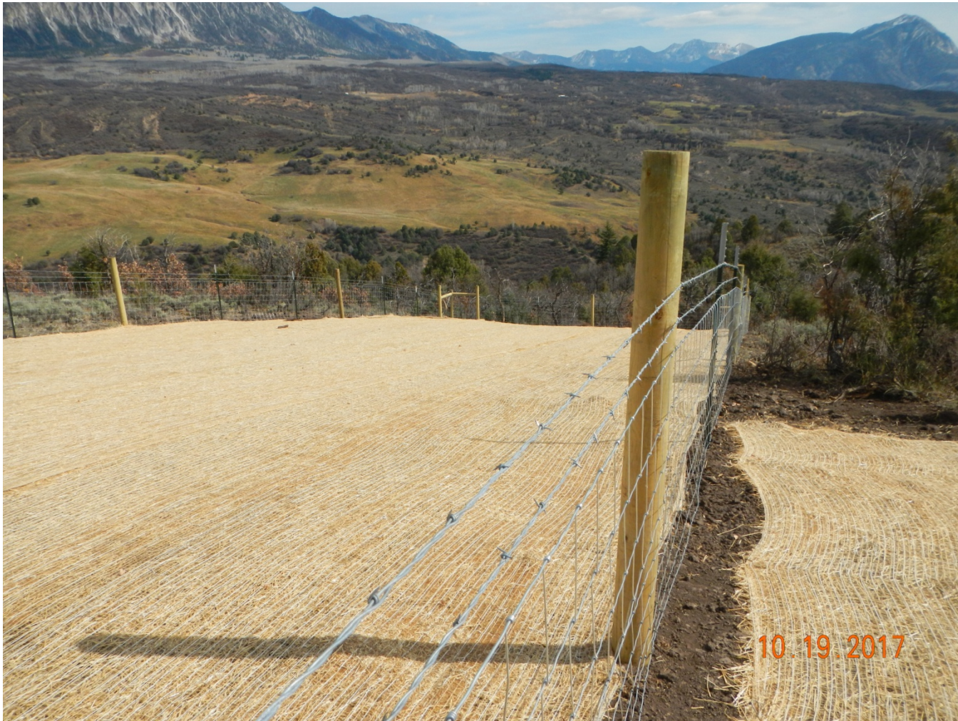
Photo 2. View of area west of repaired riser. This area is reclaimed with straw blanket and fencing.
