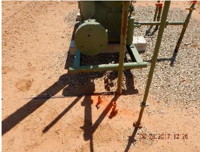
Photo 11: Risers at front of separator. Previous inspection.
