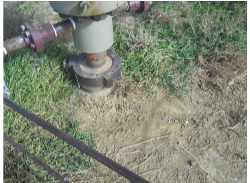
Stained soil under master valve has been cleaned up
