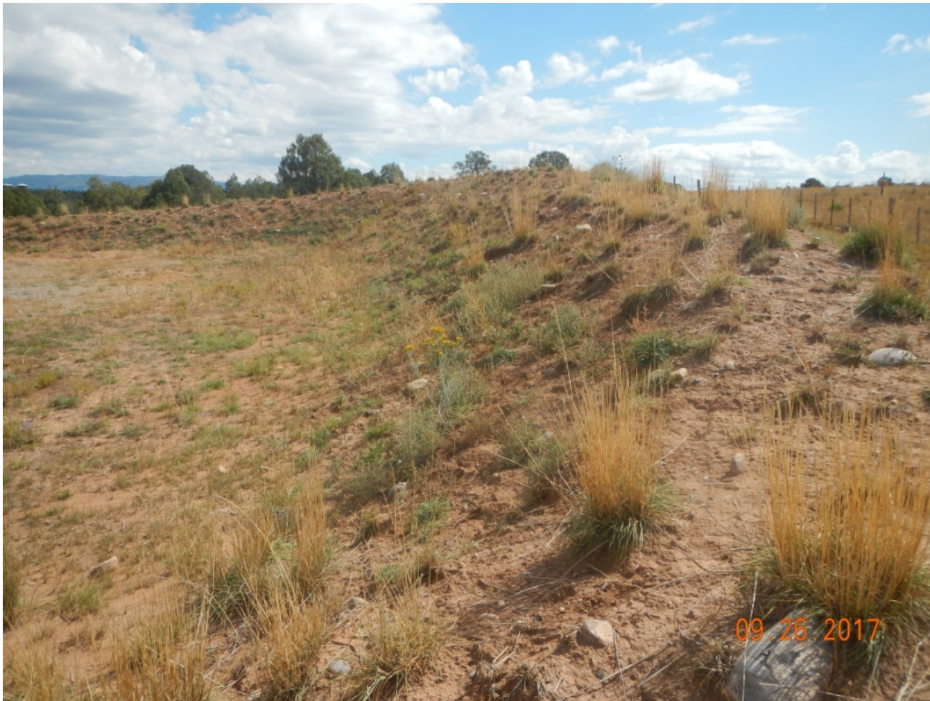
Photo 2. View of the southern portion of the project area from the southwestern corner facing eastward. Revegetation is progressing with grasses and shrubs such as crested wheatgrass ( Agropyron cristatum ), dropseed ( Sporobolus sp.), and fourwing saltbush ( Atriplex canescens ).
