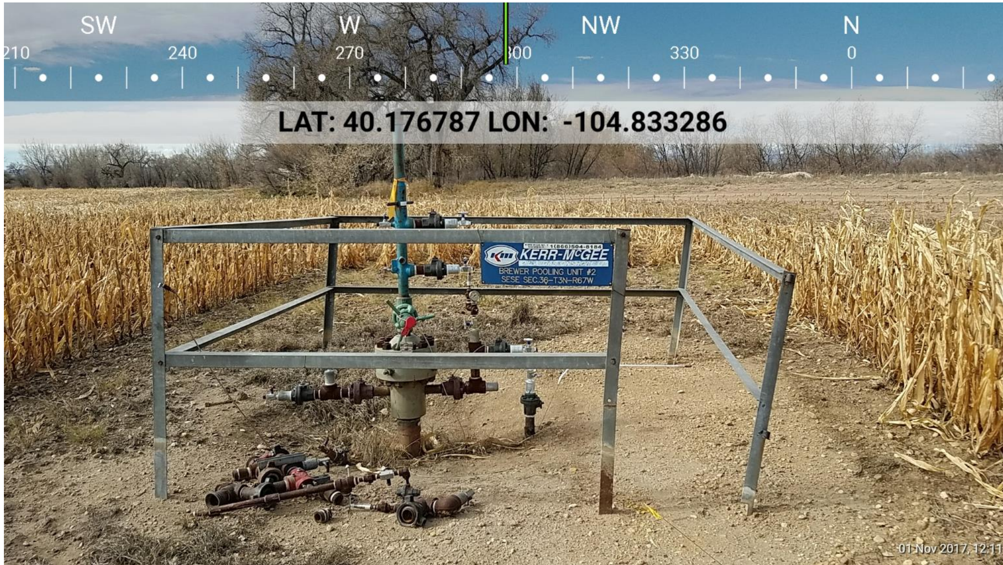
Wellhead API 05-123-10915 Location: 319237
