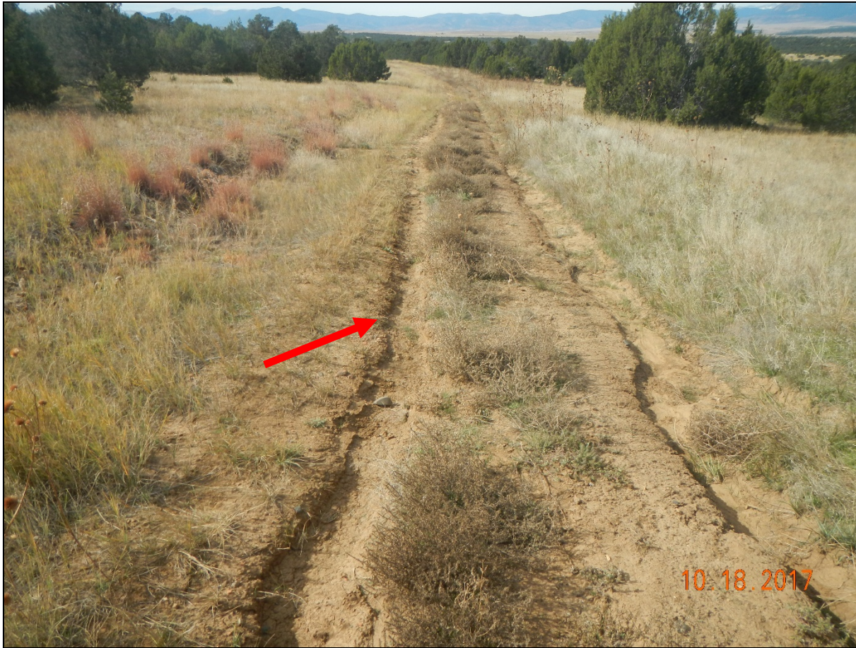
Photo 1. Facing southwest along the access road. There are signs of erosion occurring down the road.
