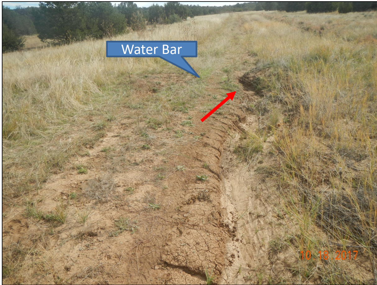
Photo 3. There is a water bar installed at this point in the road however, stormwater has eroded thru the water bar and down the road.
