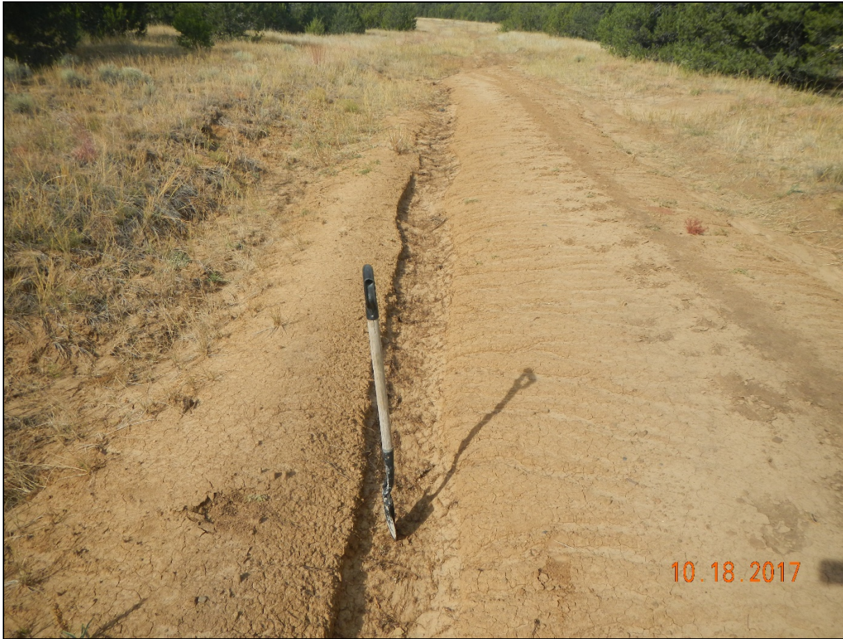
Photo 2. Facing northwest along the access road. There is stormwater erosion occurring along the road. A 3.5 ft. shovel is placed into the erosion rill for scale.
