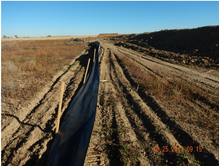
Photo 11. Photo taken from the western location, facing North. Silt fence BMP in need of maintenance.
