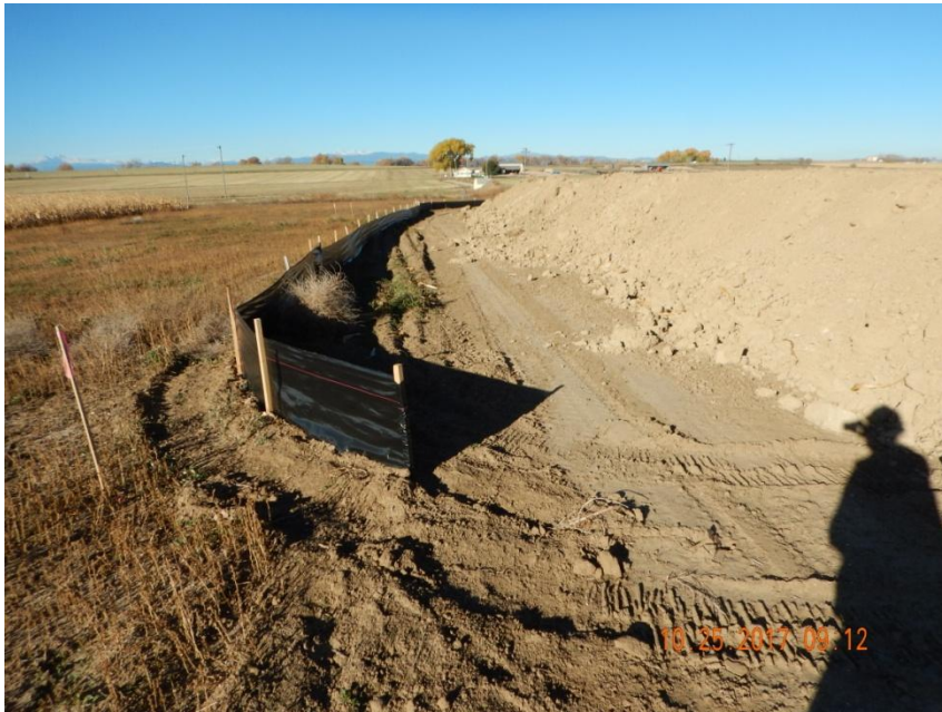
Photo 7. Photo taken from the southwestern location, facing West. Silt fence BMP has been installed along the southwest, west, and northwest perimeter of location. Fill slopes need to be stabilized.
