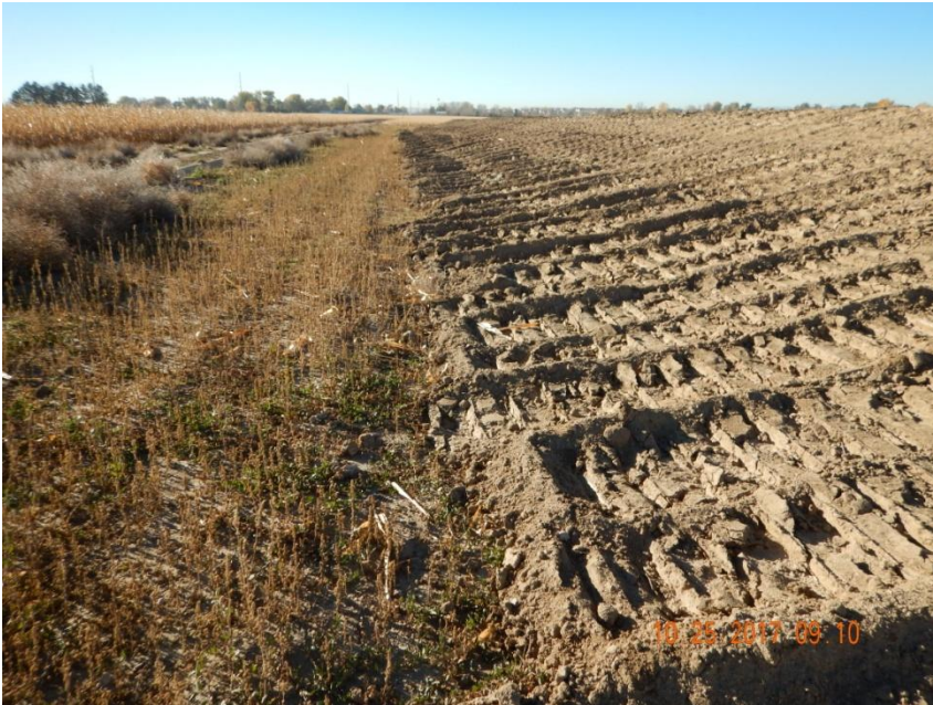
Photo 5. Photo taken from the eastern location, facing South. No stormwater and erosion control BMPs observed along the outer perimeter of stockpile.
