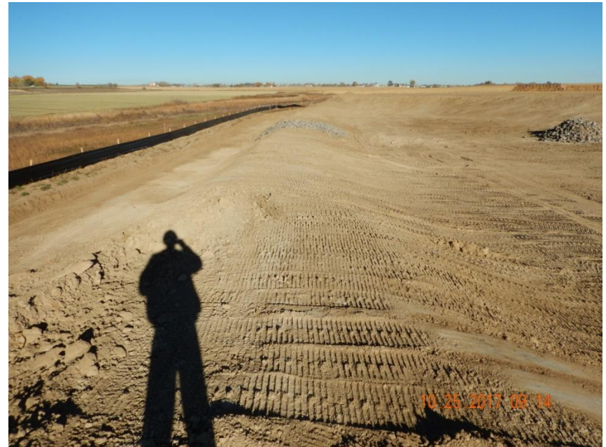
Photo 8. Photo taken from the southwestern location, facing North. Sediment basin has been constructed in conjunction with a silt fence BMP.
