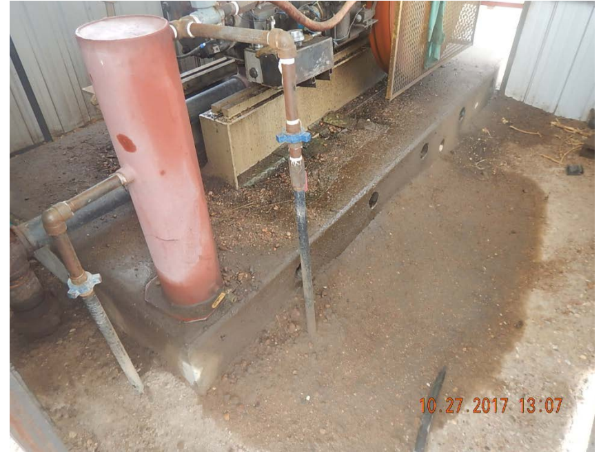
Photo 4: Stained soil at engine
