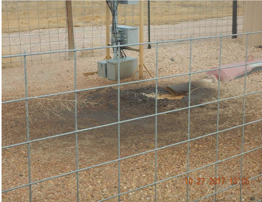
Photo 3: Stained soil at exhaust
