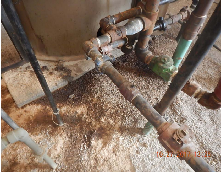
Photo 5: Stained soil in treater house
