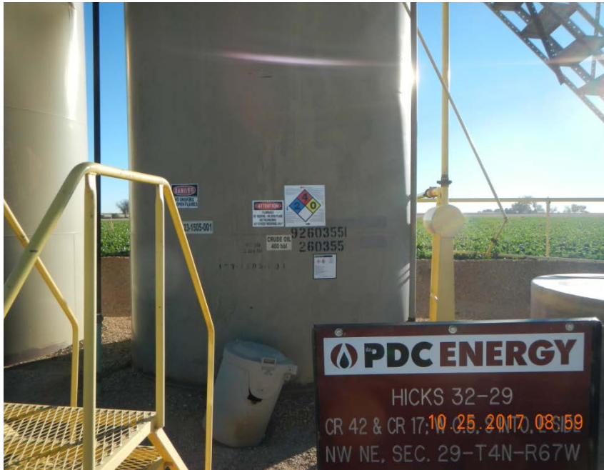
Crude oil tank placards
